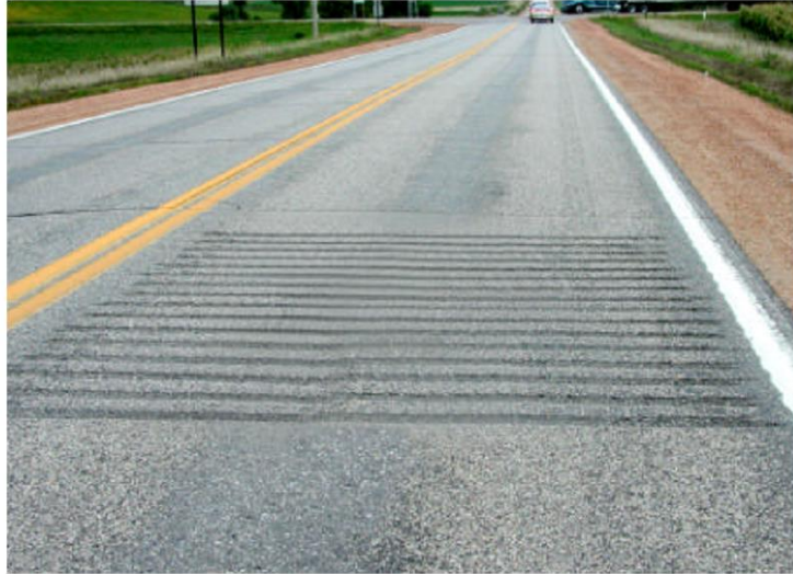
Figure 4.8: Full width rumble strip
