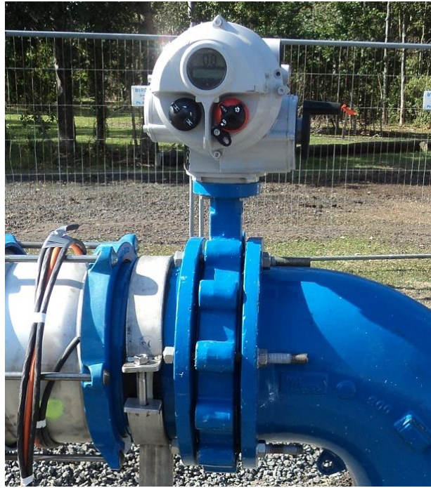
Figure 2-5 - Actuated Control Valve (Site: Water Wheels)
