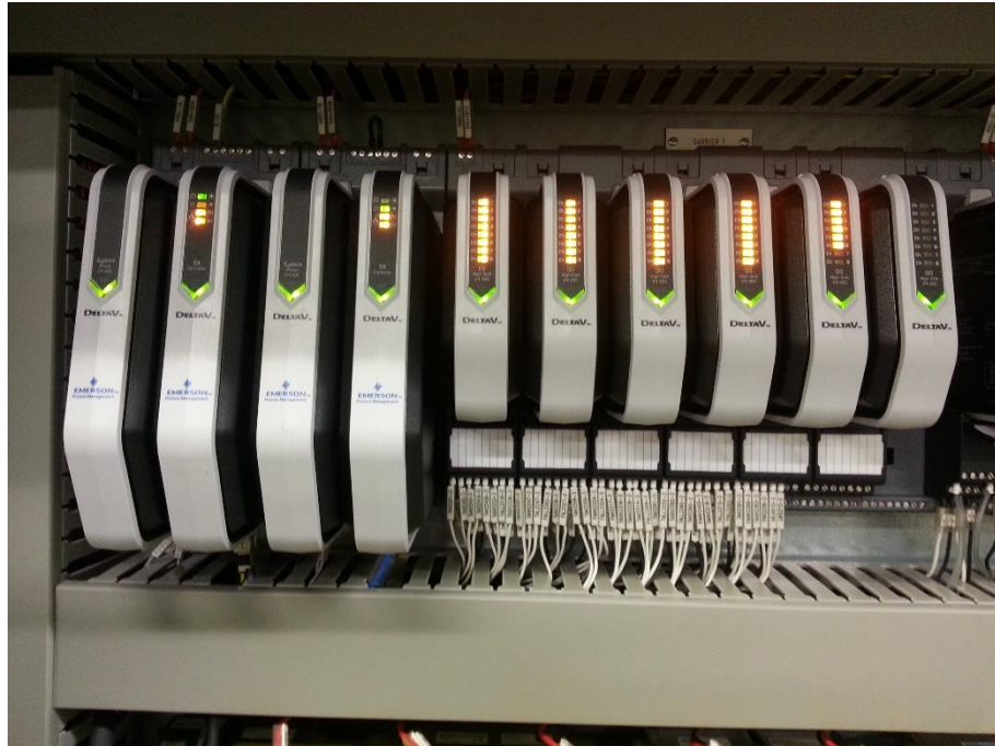
Figure 9 – Backplane mounted DCS controllers
