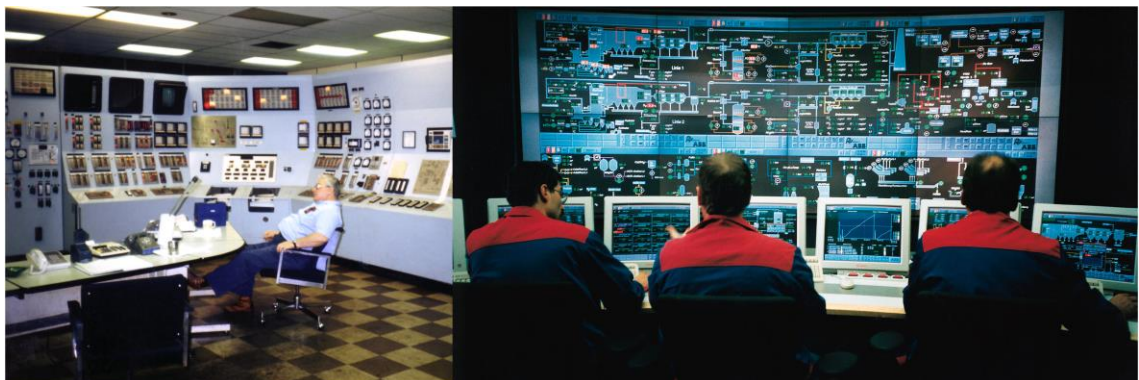
Figure 2 – Early (left) and modern (right) central control room
