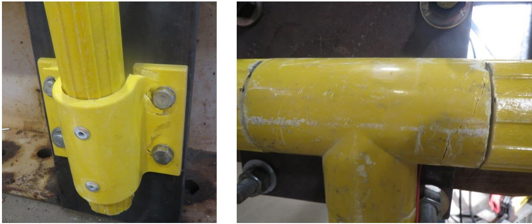
(a) Failure of the side mount plate (b) Failure of 3-way tee at the top post
