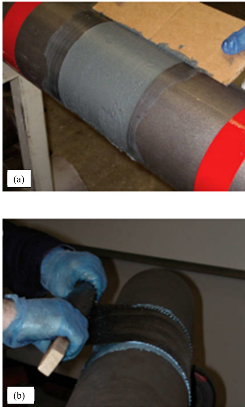
Figure 2.6 Pipe exterior repair process using infill and flexible wrap (a) Filling defect with putty (b) Wrapping epoxy wetted carbon fabric around the defect (Duell et al. 2008)
