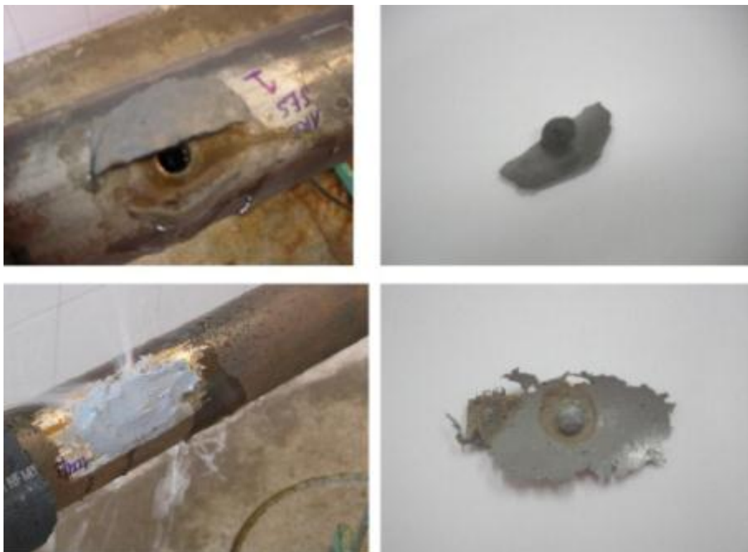
Figure 2.13 Failure of epoxy repair (Mattos et al. 2012)
