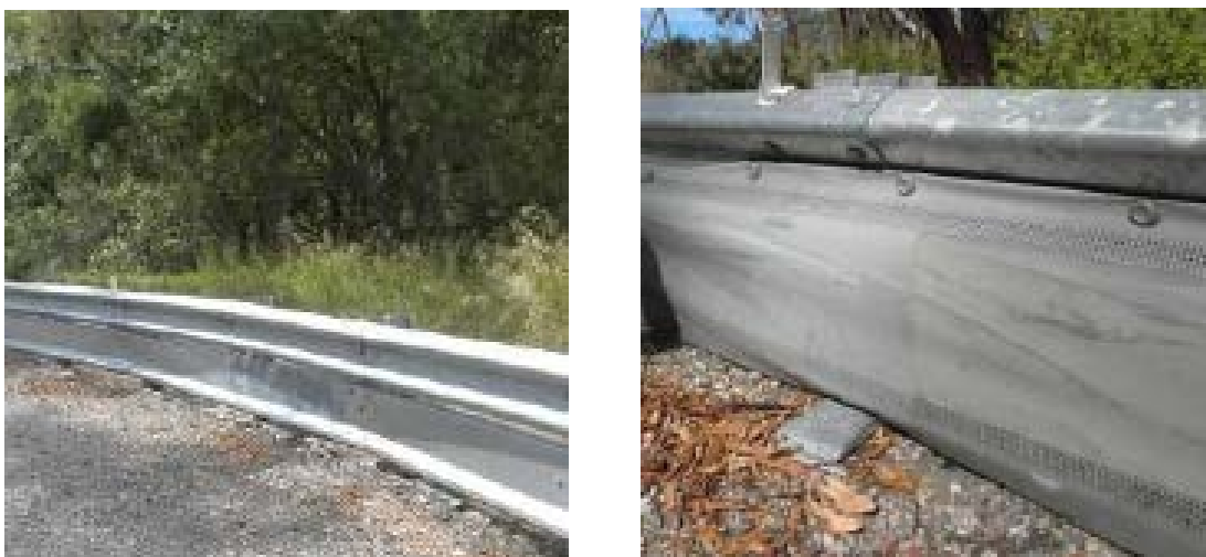
Figure 4 – W-beam retrofitted with rubrail and flexible mesh (Anderson et al, 2012)
