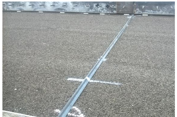
Step 6– Installation of triangle crack inducers on bottom and sides of slab.
