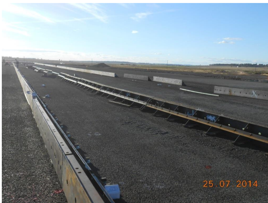
Figure 47 - The run in the middle is currently supporting the formwork for the runs either side. Once each side is completed and the formwork is removed the middle run will be paved as an infill run.
