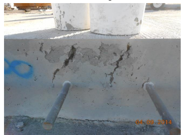
Photo 2 – Air voids extending into slab.
