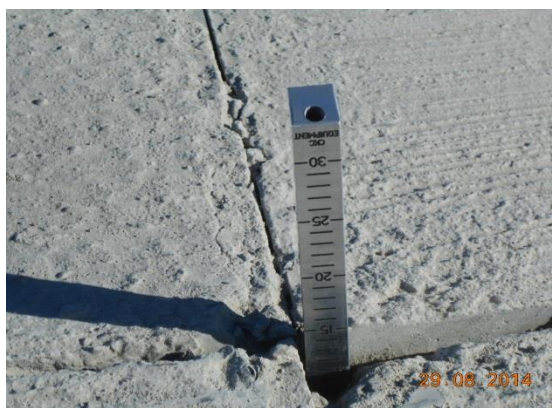
Photo 1 - Spalling between concrete slabs.
