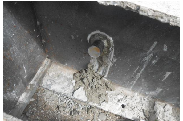
Photo 6 – Collar vibrated off dowel bar which has fallen into the pour.
