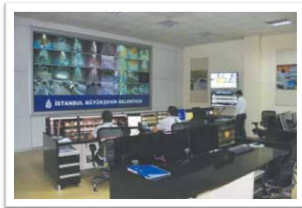
Figure 20 - Example of tunnel control room
