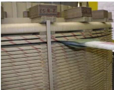
(a) Paper insulation wrapped around transformer windings.
