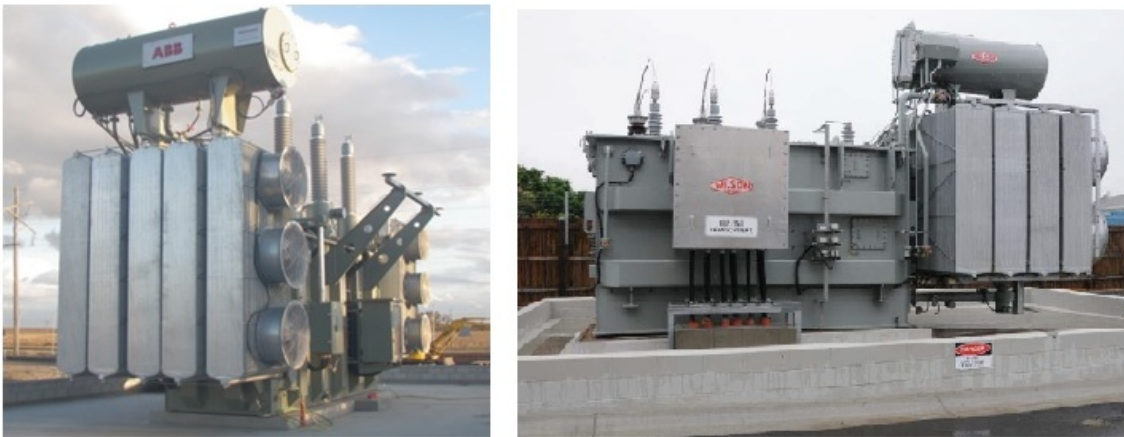
Figure 1.1: Typical power transformers ( Source: G.Caldwell, Ergon Energy ).
