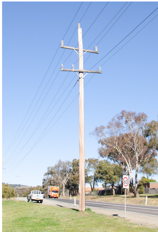
Figure 4.1: Pole CE19317 located at Cooma Street, Queanbeyan
