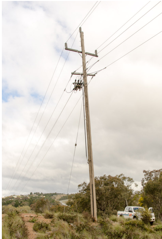
Figure 4.15: Pole CE19321 located at Old Cooma Road near Queanbeyan
