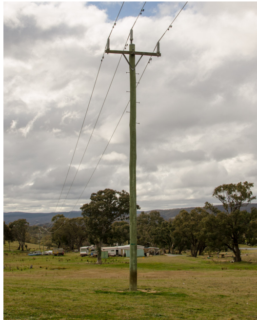
Figure 4.19: Pole CE69899 located at Quarry Road near Queanbeyan
