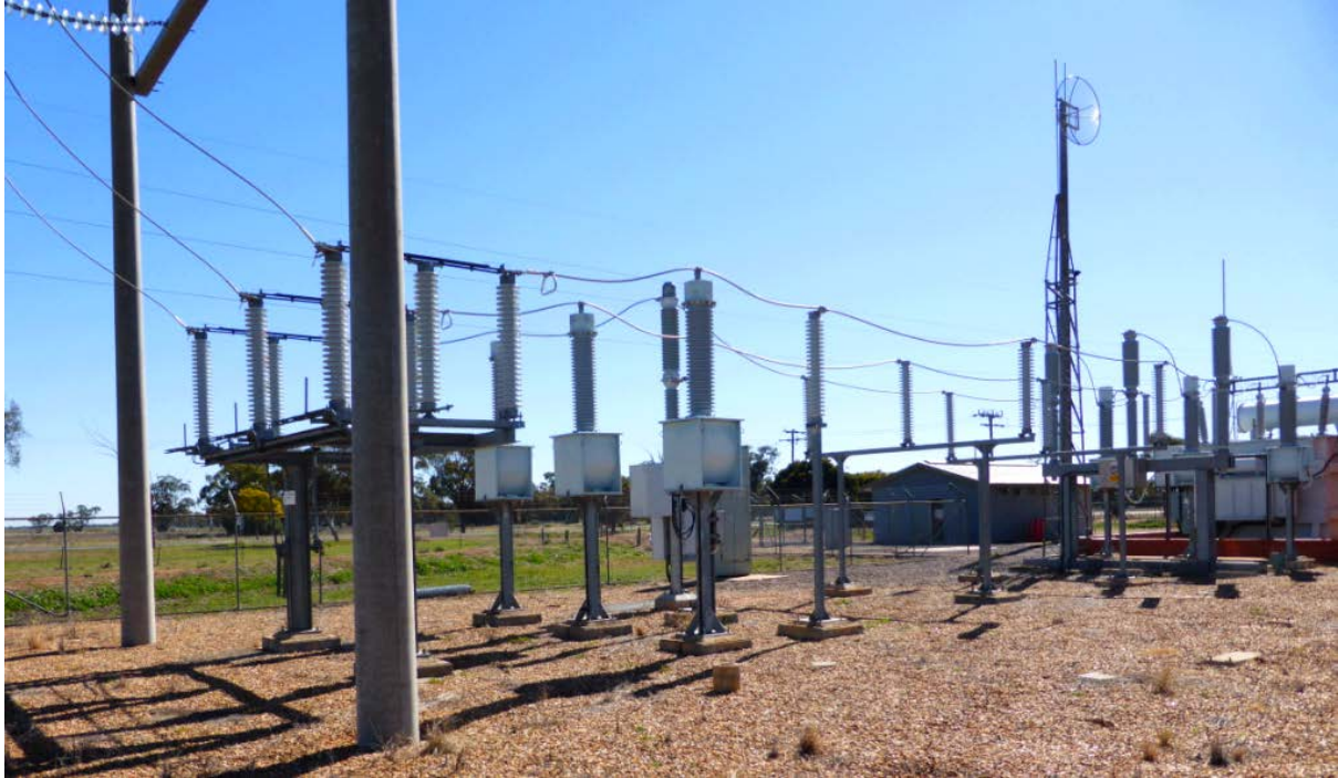
Figure 27: Nevertire 132kV feeder bay circuit breaker 4422
