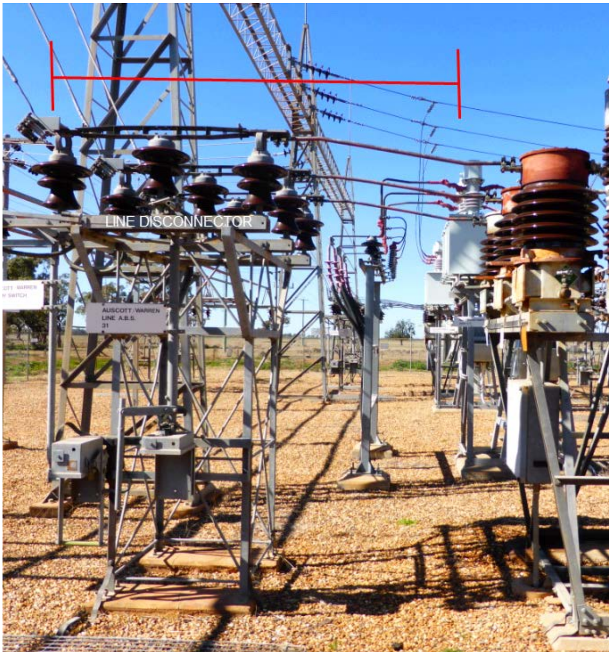
Figure 49: Circuit breaker 32 line side section safety clearance.
