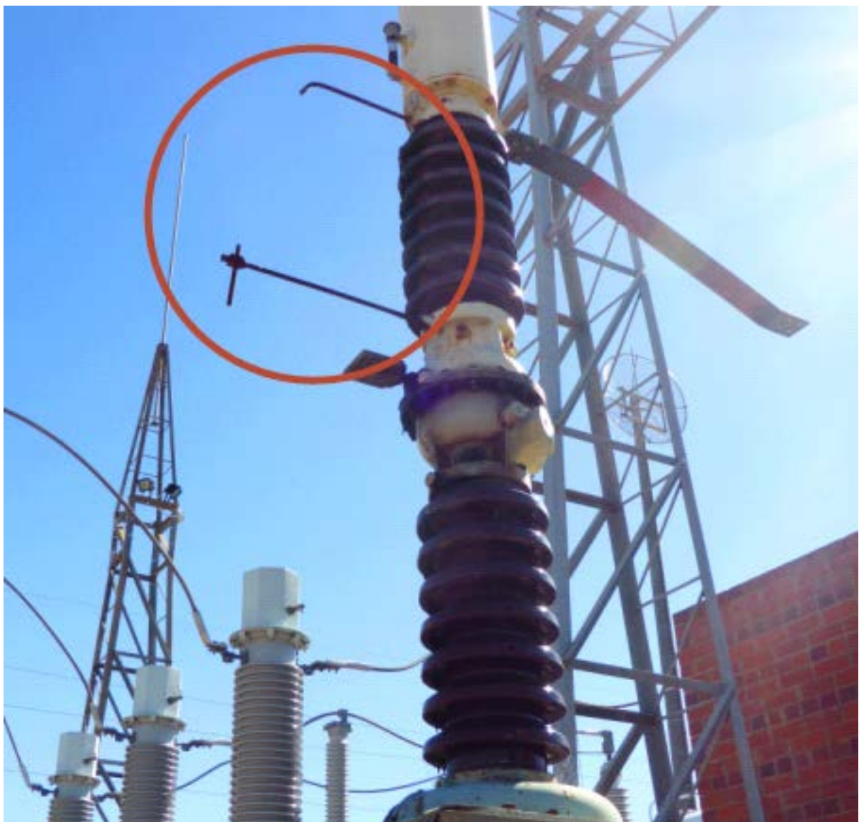
Figure 9: Spark gap shown on spare single pole circuit breaker.
