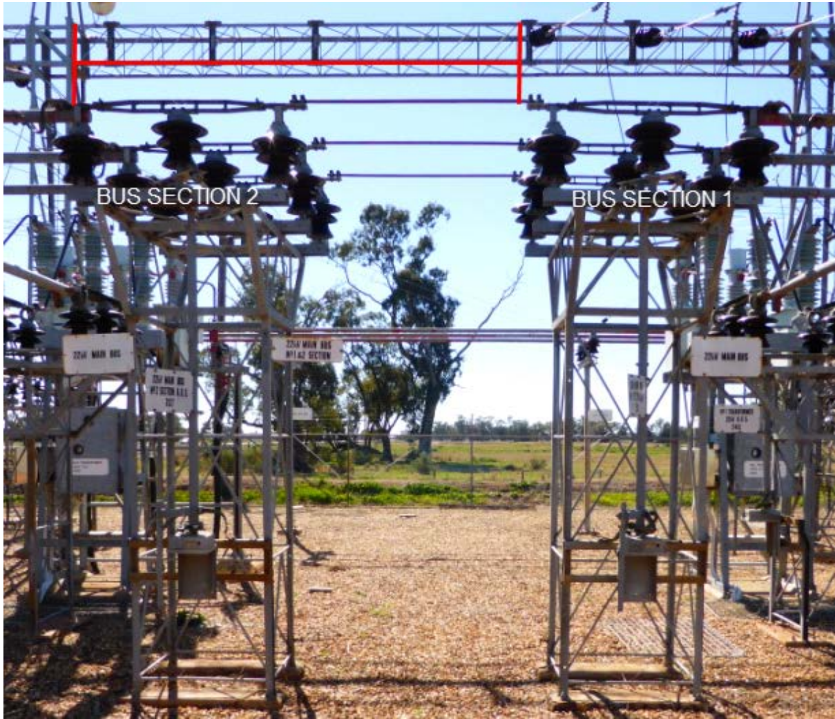
Figure 45: 22kV Main busbar disconnectors section safety clearance.
