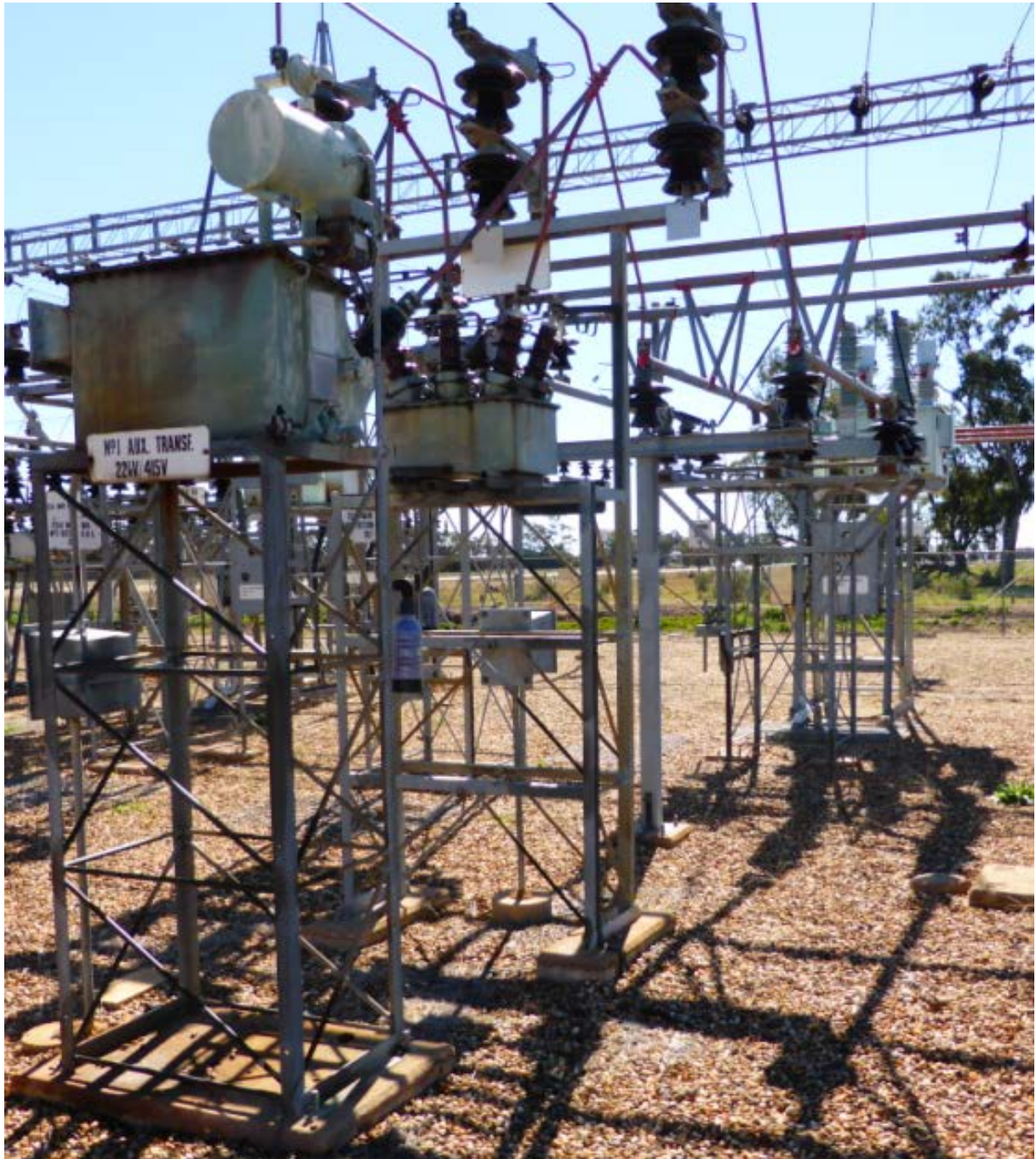
Figure 38: 22kV Transformer circuit breaker 2412.
