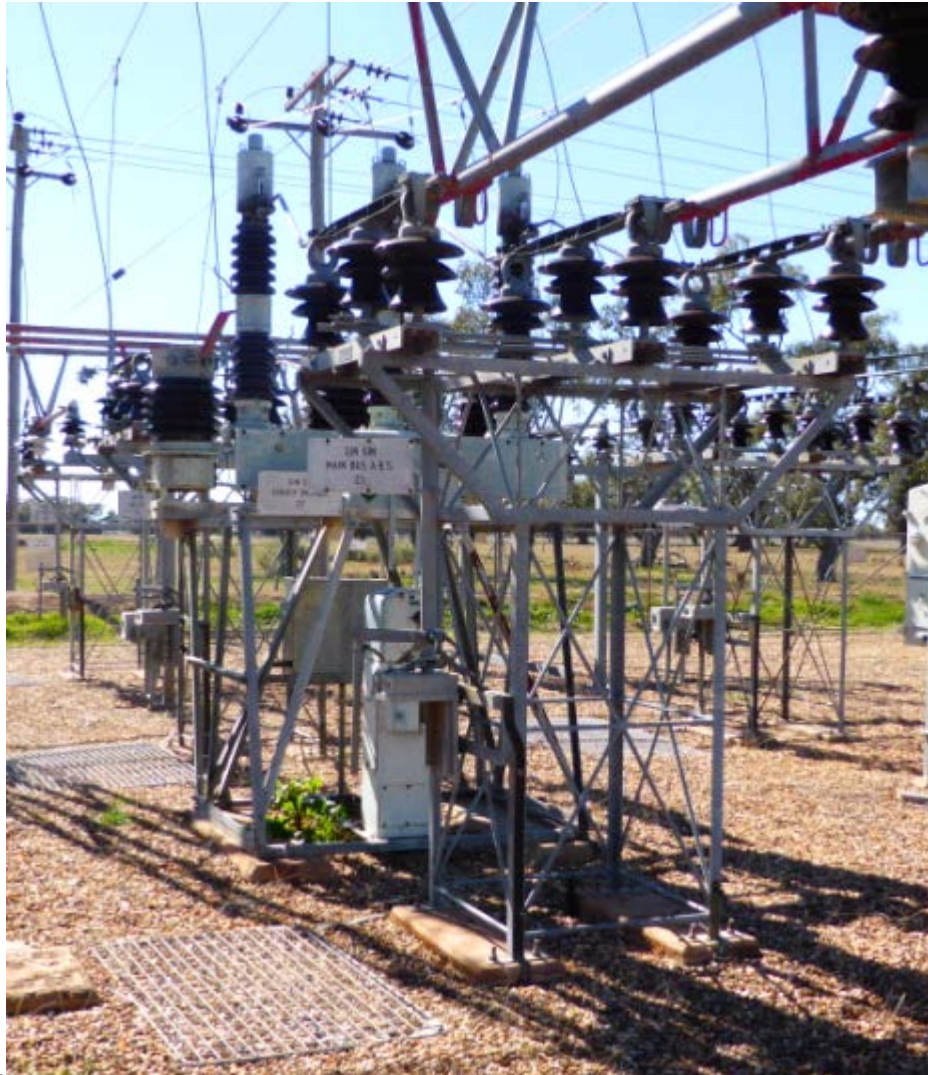
Figure 34: 22kV Feeder bay circuit breaker 22.
