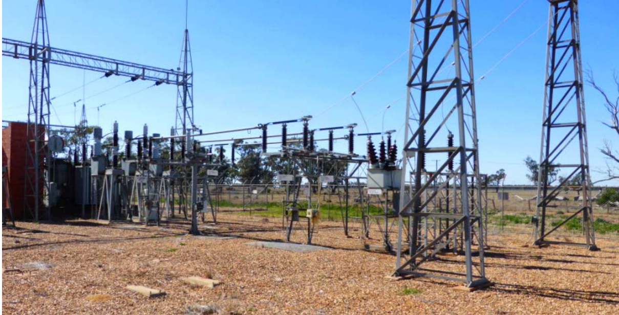
Figure 28: Nevertire 66kV feeder bay circuit breaker 3412.
