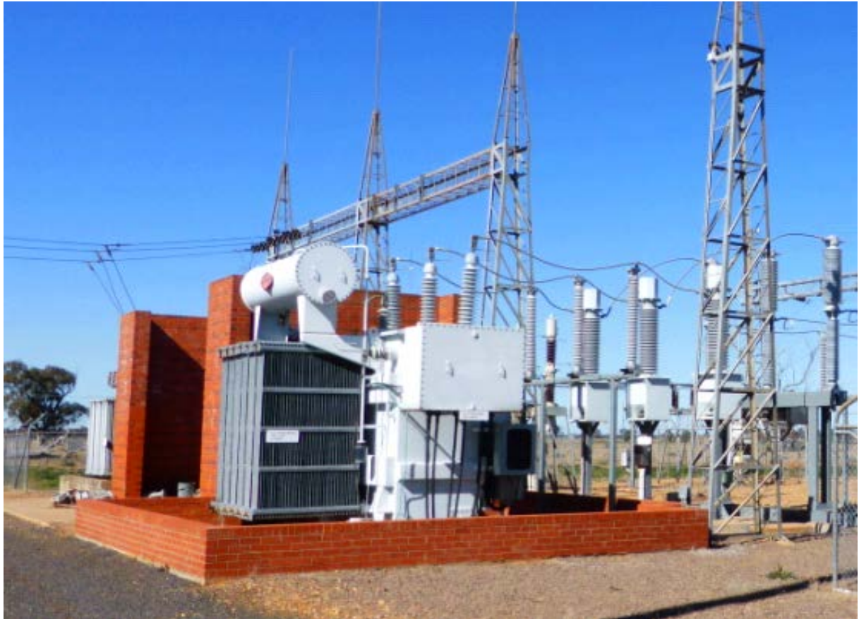
Figure 22: Item 14 132kV transformer front and side bund wall.
