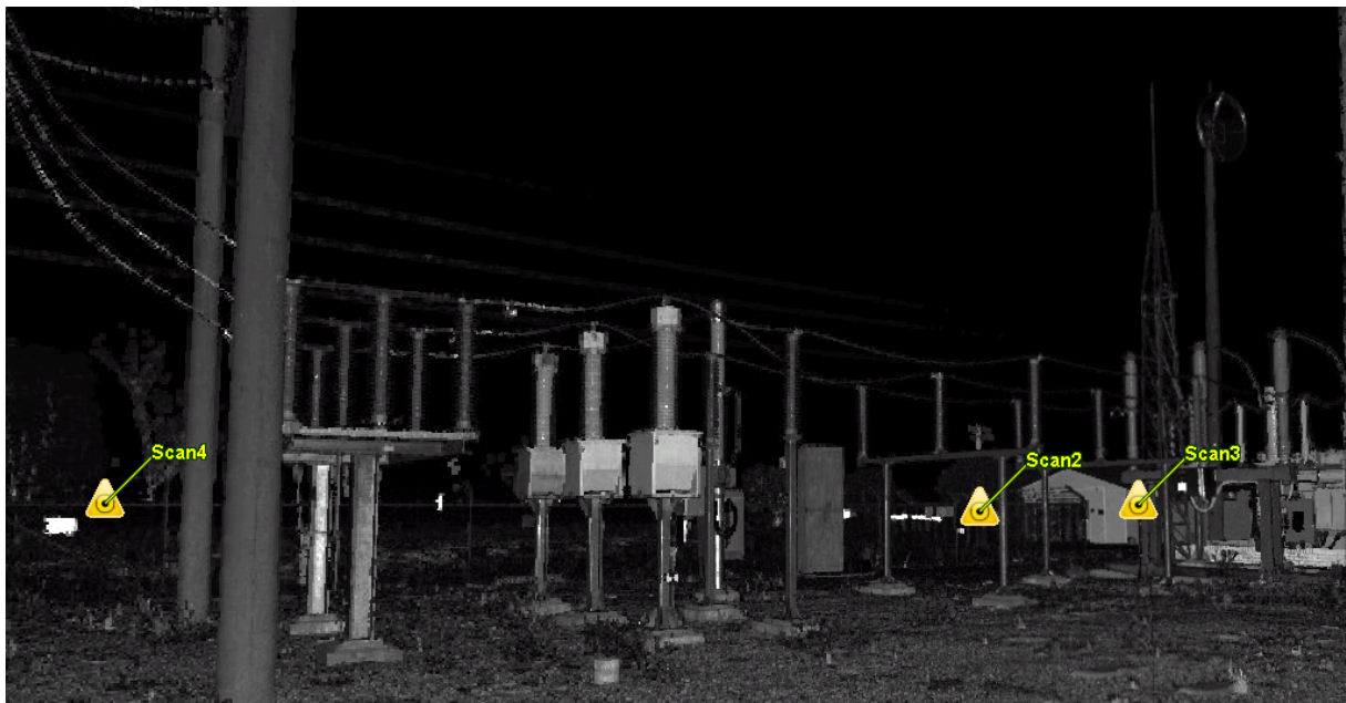
Figure 26: Leica TruView file screen shot displaying 132kV feeder bay.
