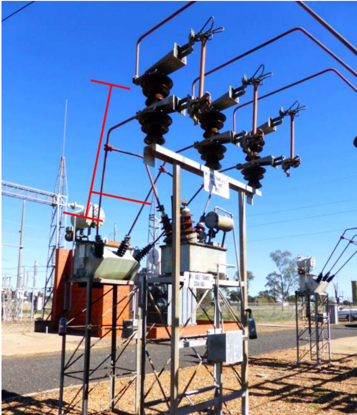
Figure 40: No.1 22kV/415V Aux. and VT section safety clearance.
