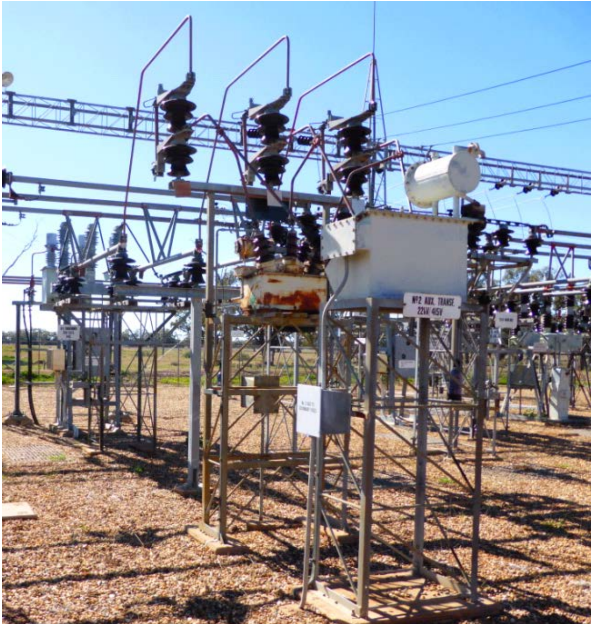
Figure 42: 22kV Transformer CB 2422 and No.2 22kV/415V Aux. and VT.
