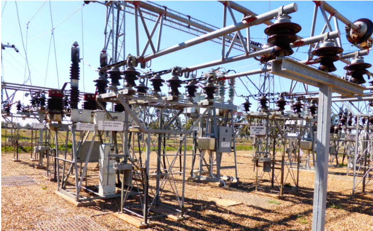
Figure 46: 22kV Feeder bay circuit breaker 32.
