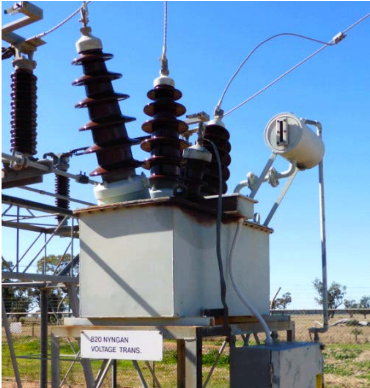
Figure 30: 66kV feeder bay voltage transformer.
