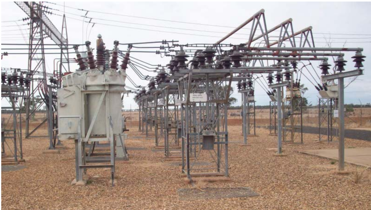
Figure 4: 22kV Substation equipment with suspected poor clearances.
