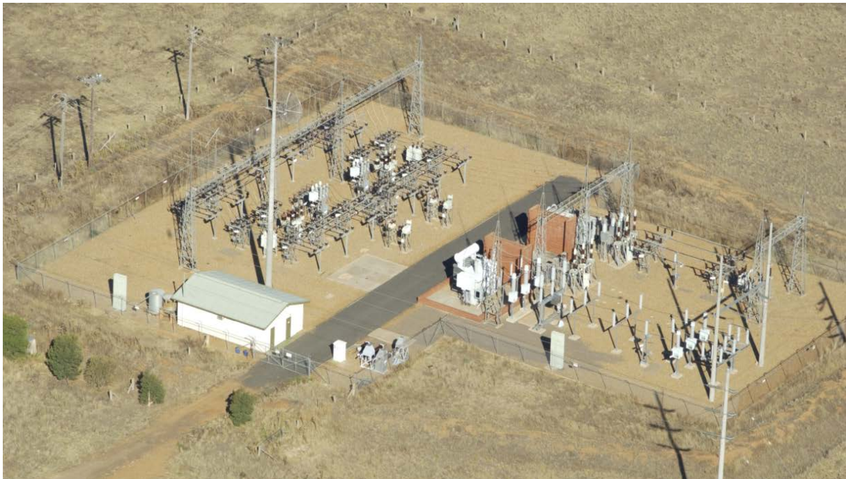
Figure 3: Nevertire Zone Substation site overview.
