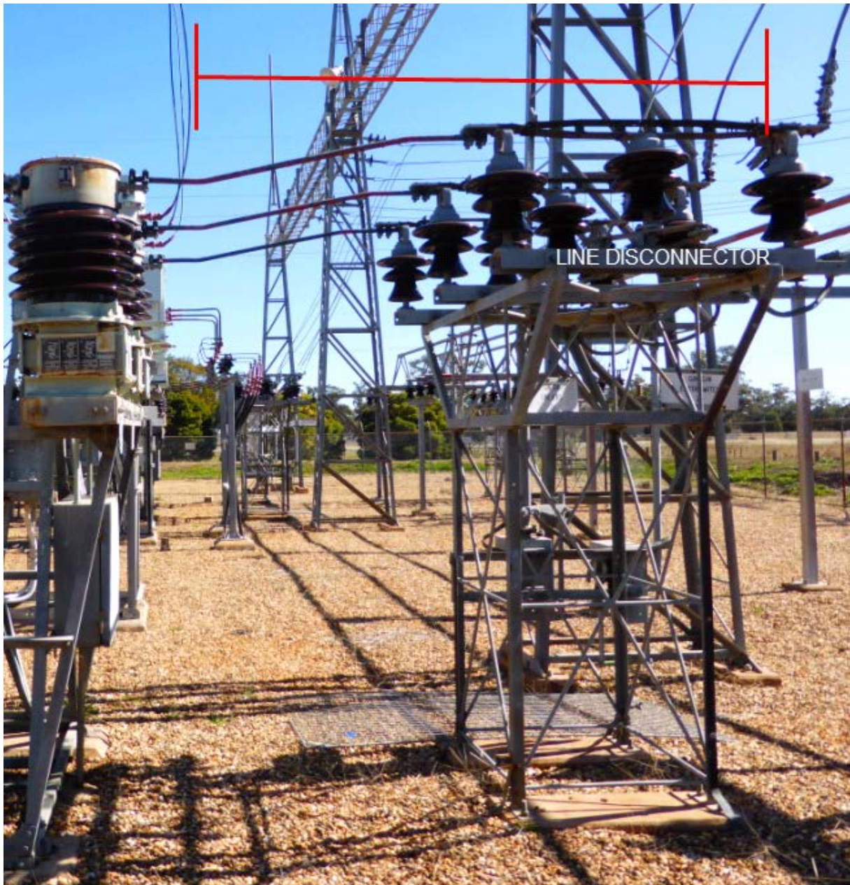
Figure 37: Circuit breaker 22 line side section safety clearance.
