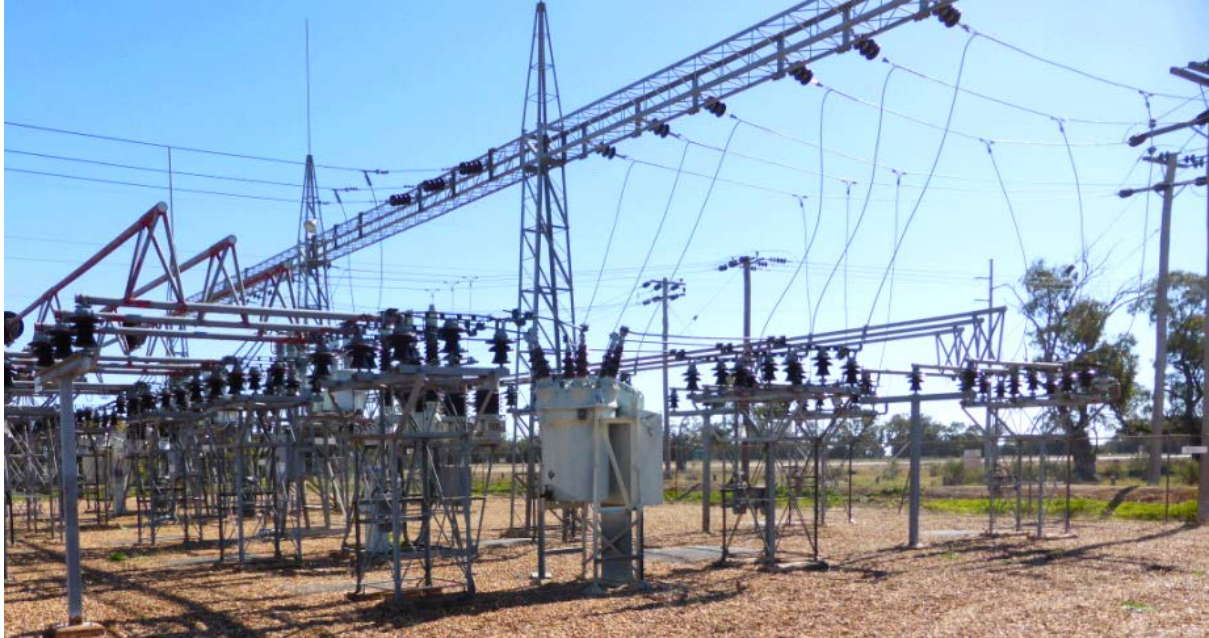
Figure 31: 22kV Feeder bay circuit breaker 12.
