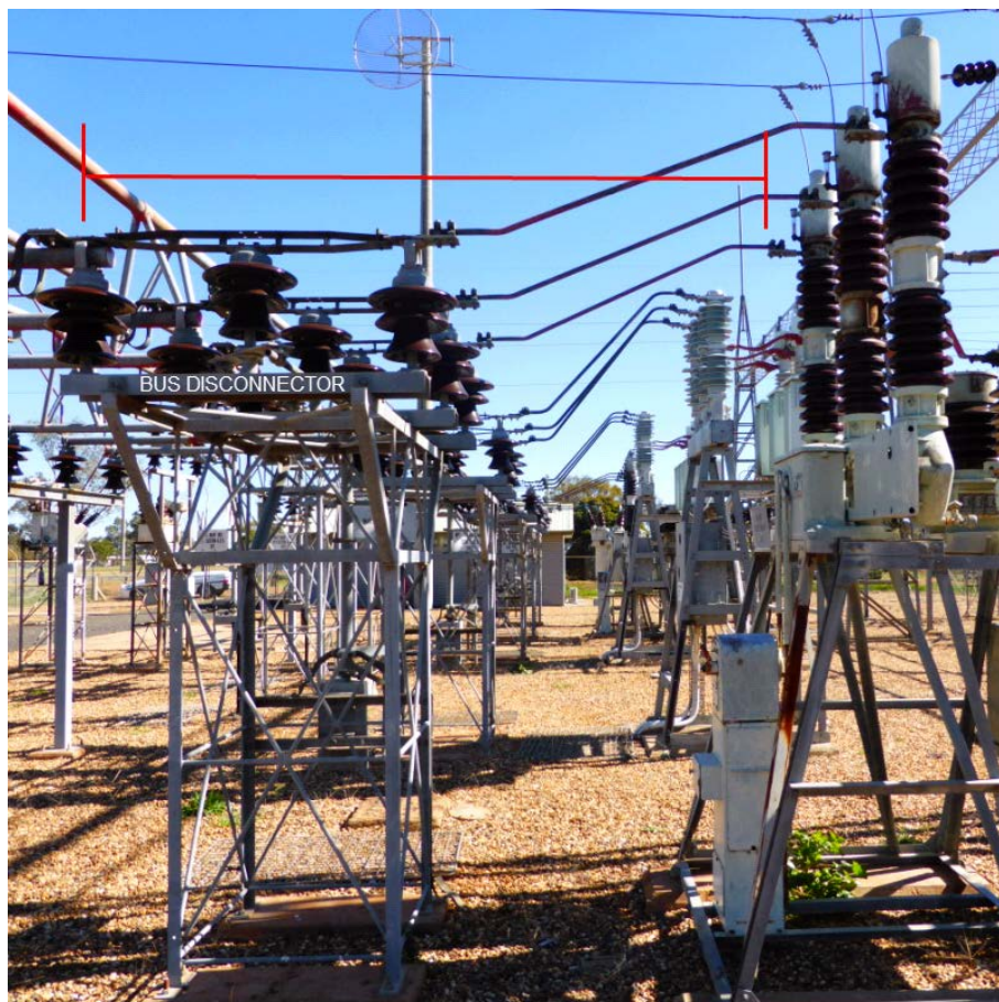
Figure 36: 22kV Circuit breaker 22 bus side section safety clearance.
