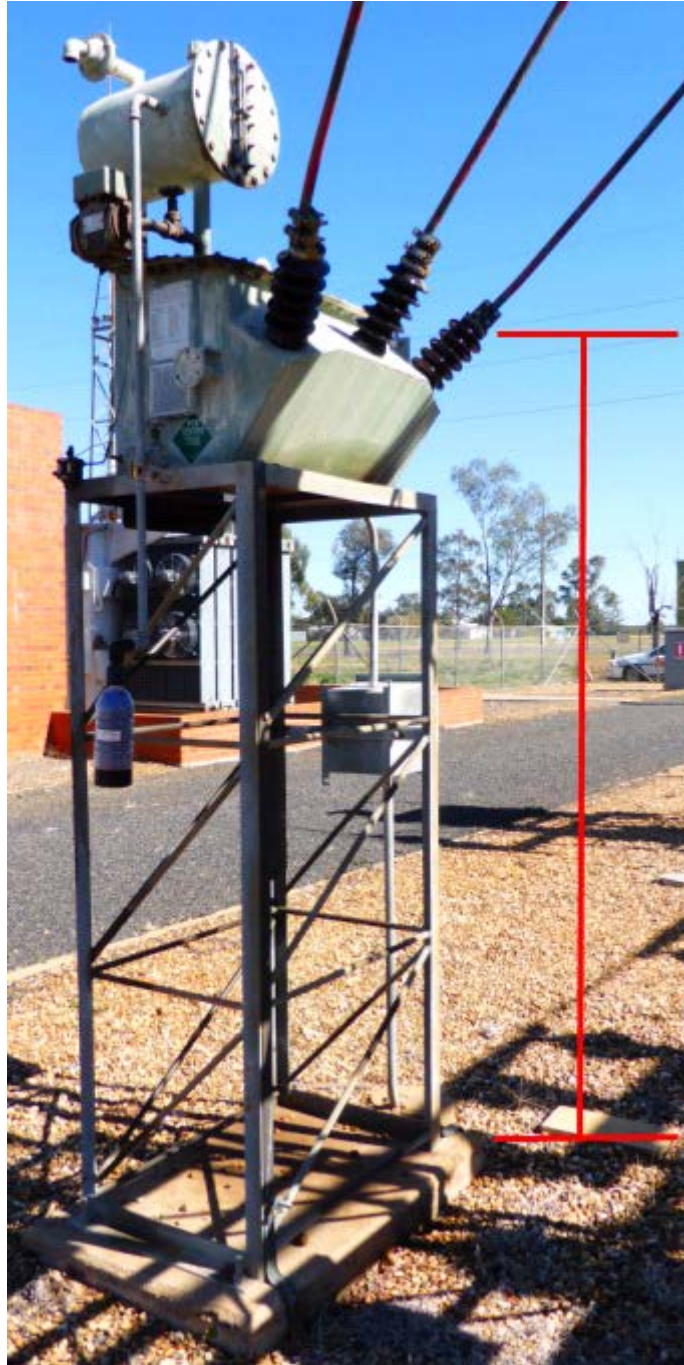
Figure 39: No.1 22kV/415V auxiliary voltage transformer.
