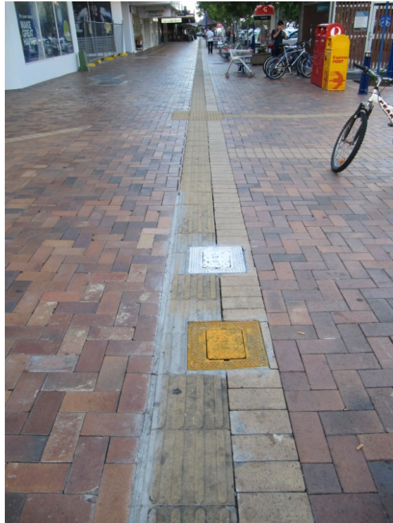
Figure 4.30(b) – Lids to underground services interrupt the tactile surface path for the vision impaired
