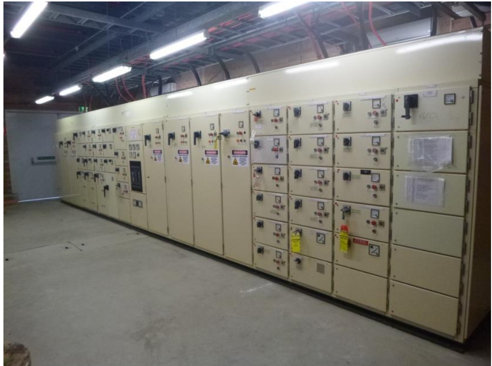
Figure 2-3: MCC P6512 - Located in EDC K4
