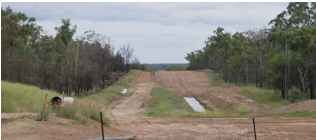
Figure 6: CSG gathering line right of way demonstrating limited vegetation establishment and subsidence.
