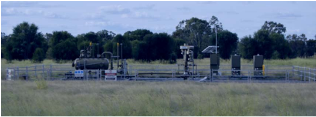
Figure 7. Fenced off operational CSG well pad (~12 x 8 m, initial construction area outside fenced area) (Arrow, 2012)
