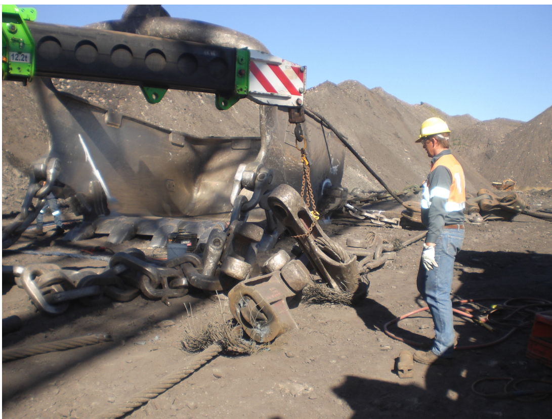
Illustration 3: Dragline rigging repair in action. Due to weight the majority of repair actions require use of a 20 ton crane for load support. Many standard rigging elements such as captive hooks are not used in rigging maintenance.
