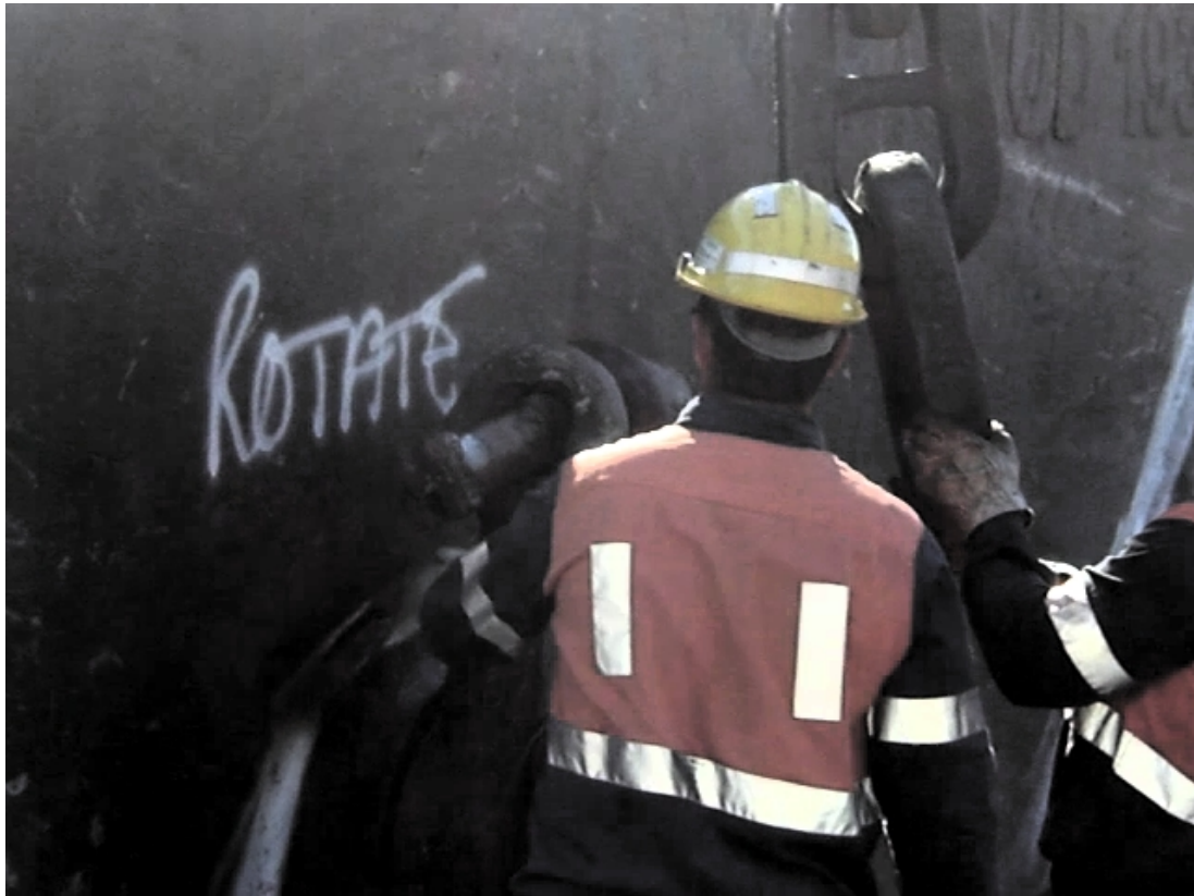
Illustration 4: Rotation of Lower Hoist Chains requires workers to be exposed to the risk of catastrophic injury in the event of a falling hoist chain.
