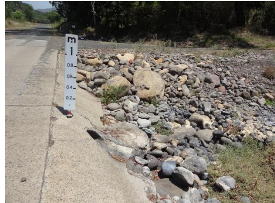
Rock protection structure damaged
