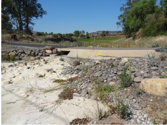
Undermined and cracked
