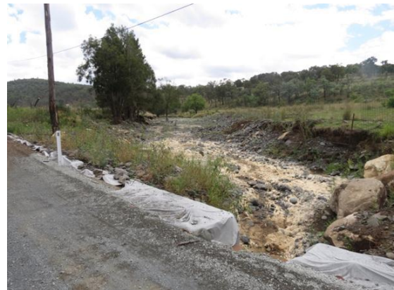
Damaged at upstream
