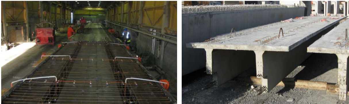
Figure 4: Sections showing instrumentation of prestressed double tee unit (top) and photographs showing installation of gauges in precasting yard (bottom).
