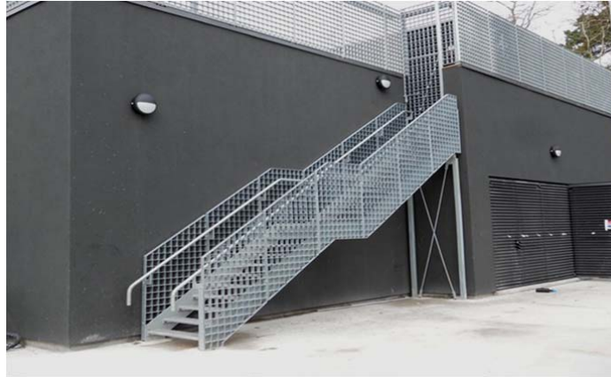
Figure 11: Lightweight steel stairs which will be used to illustrate the phenomenon of footfall induced vibrations.
