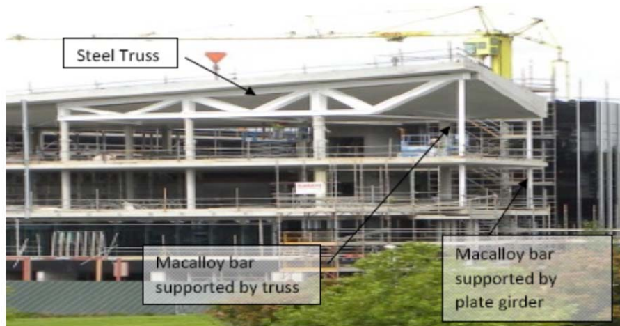
Figure 5: Image showing location of structural steel truss in south wing of the NEB.
