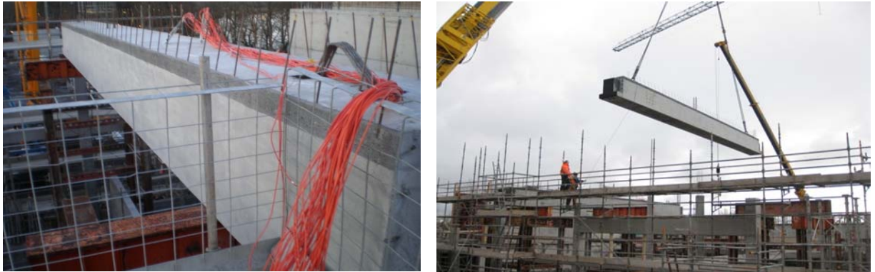
Figure 3: Sections showing instrumentation of prestressed box beam (top) and photographs showing installation of beam on site (bottom).
