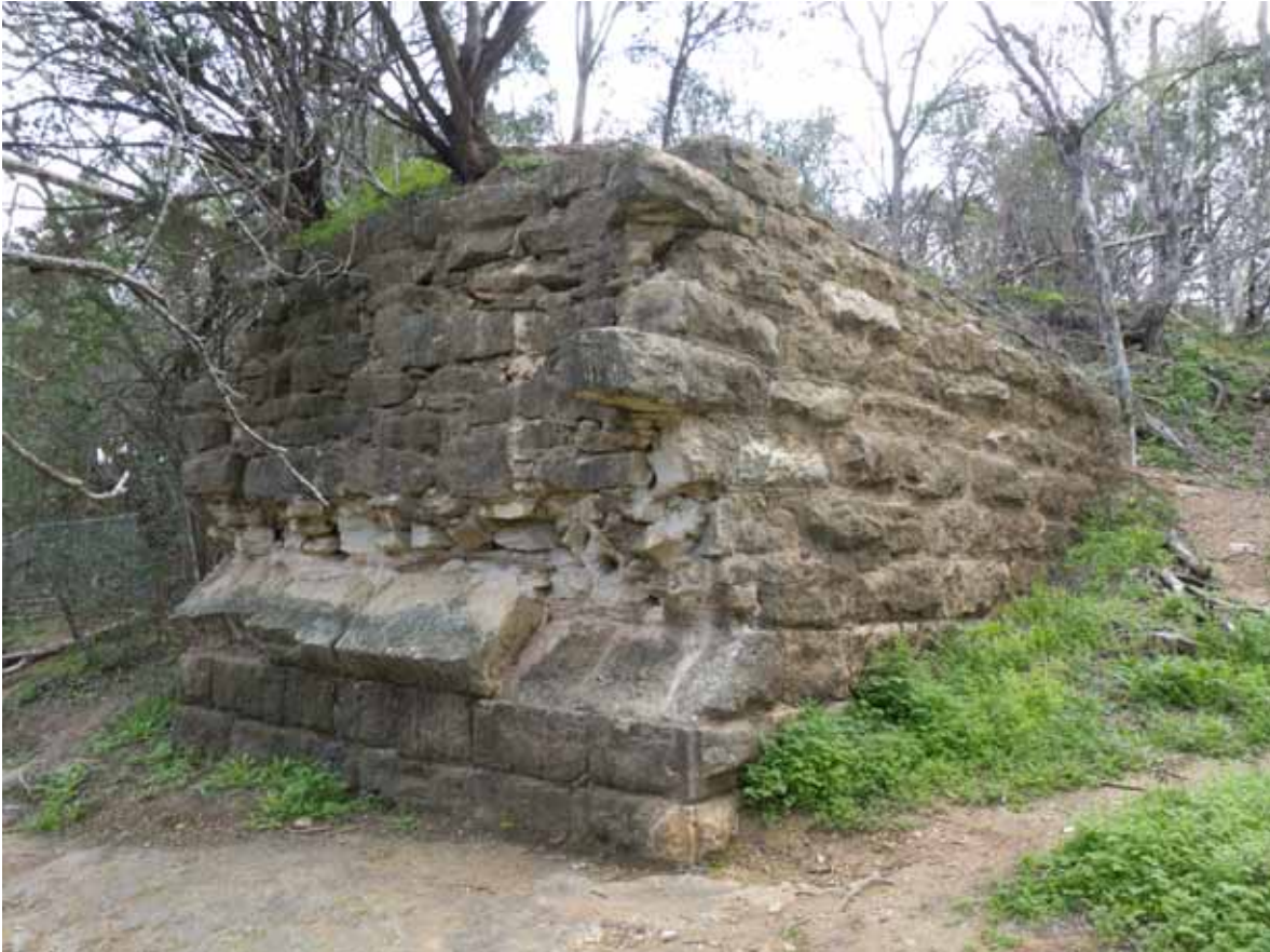
Landscape Characteristic E7 – Barton Springs Bridge Abutment: West side of the abutment, located on the south bank of Barton Creek, west of the swimming area. Facing southeast. Photograph take by Julie McGilvray, 2012.
