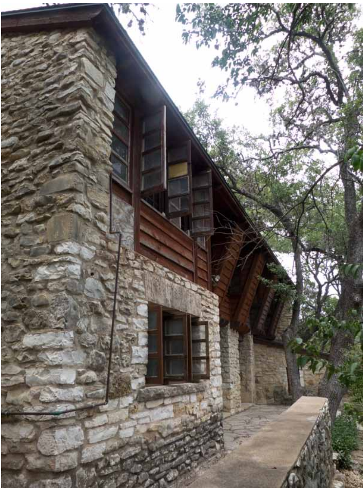
Landscape Characteristic F12 – Girl Scout Cabin: South elevation, facing west-northwest. Photograph taken by Julie McGilvray, 2012.
