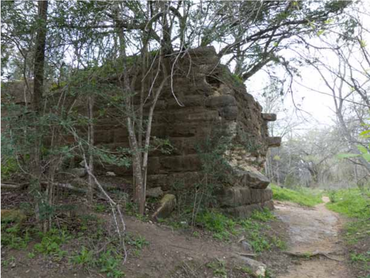
Landscape Characteristic F30 – Barton Springs Bridge Abutment: Overview of east and north face of abutment. Facing southwest.
