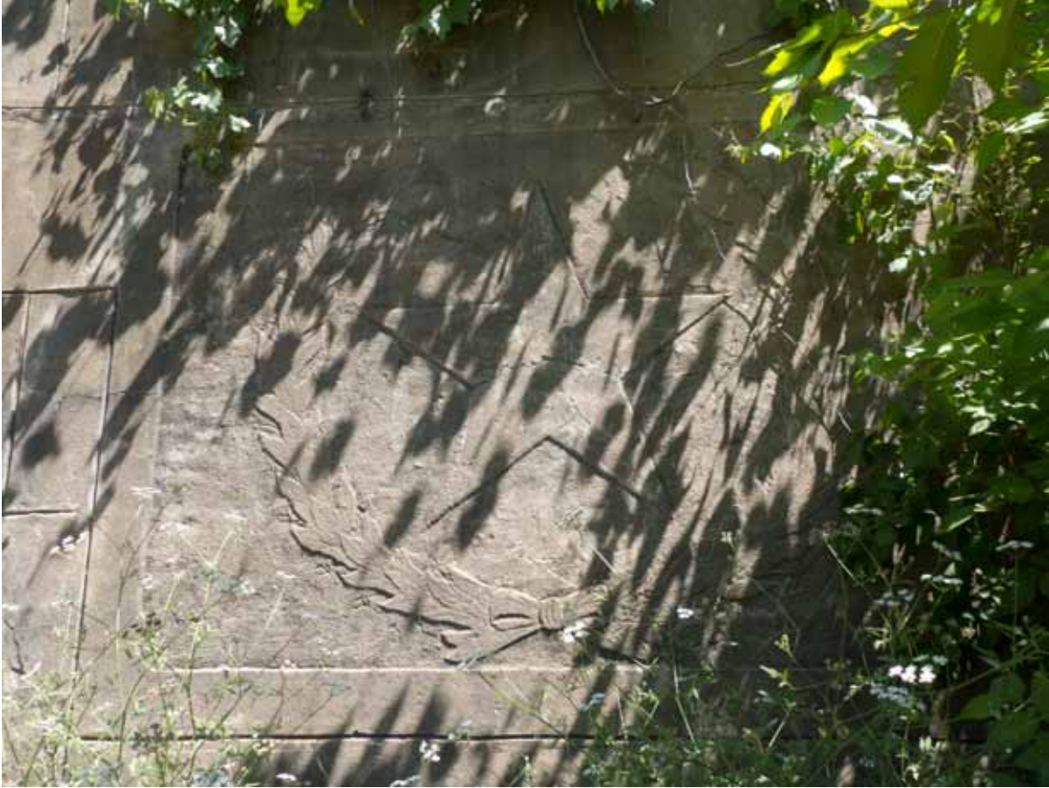
Landscape Characteristic F31 – Elk's Pit (Eliza Spring): Star motif concrete panel. Located on wall panel of pit. Facing southwest.
