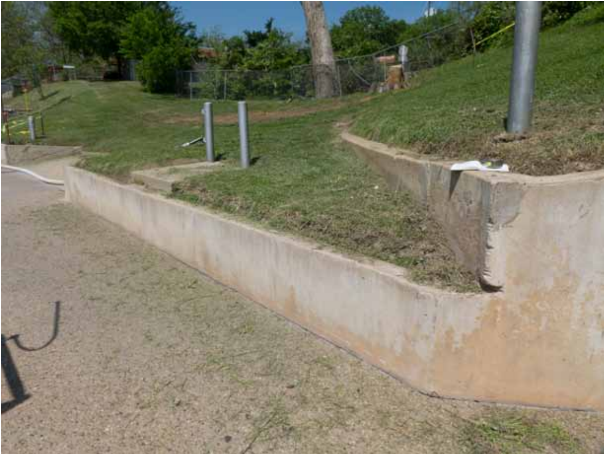
Landscape Characteristic F21 – Barton Springs Pool: Detail of concrete retaining wall system located on north bank, east end of pool. Facing northwest. Photograph take by Julie McGilvray, 2012.
