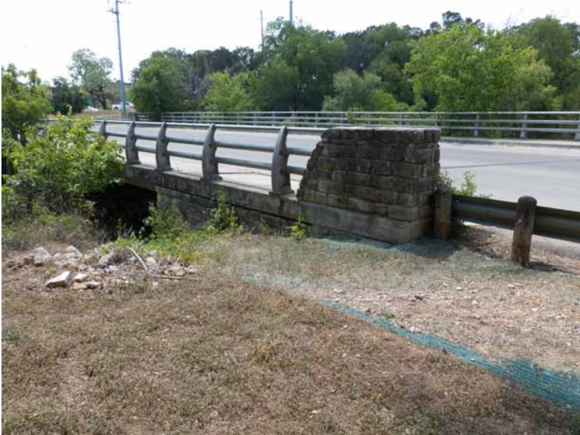
Landscape Characteristic F7 – Rollingwood Bridge Abutment: View of northwest abutment. Facing southeast. Photograph taken by Julie McGilvray, 2012.
