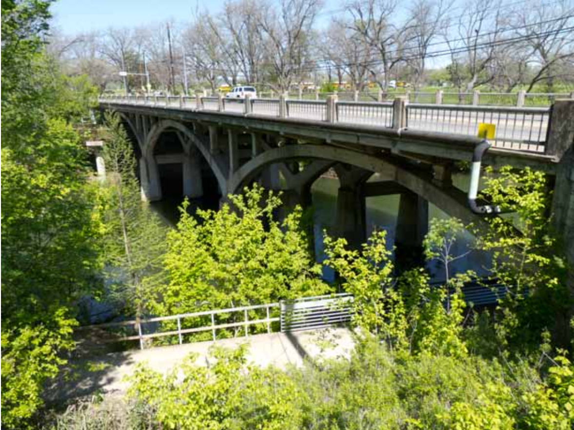
Landscape Characteristic F1 – Barton Springs Road Bridge: Overview of bridge from the south bank of Barton Creek at Barton Springs Road/Robert E. Lee Road intersection. Facing northwest. Photograph taken by Julie McGilvray, 2012.
