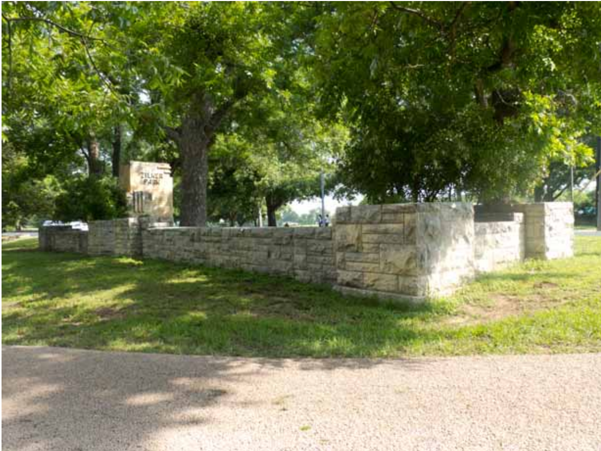
Landscape Characteristic F2 – Zilker Park Entry Gateway on Barton Springs Road: Overview of gateway structure located on the southwest side of Barton Springs Rd. Facing north-northwest. Photograph taken by Julie McGilvray, 2012.
