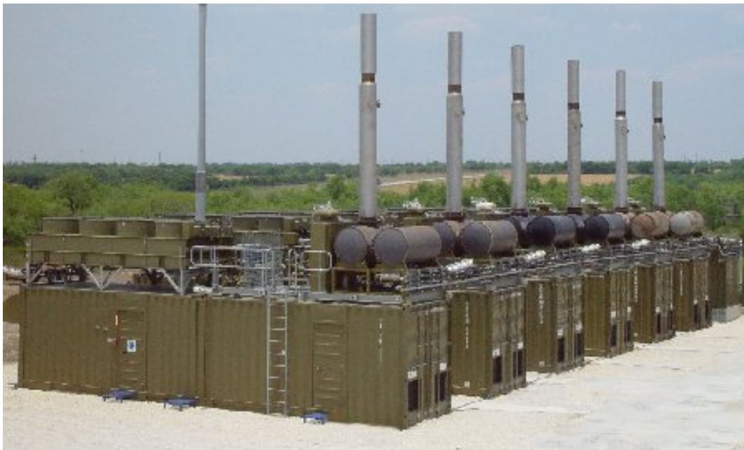
Figure 13.11 Landfill Gas-to-Energy Power Plant
