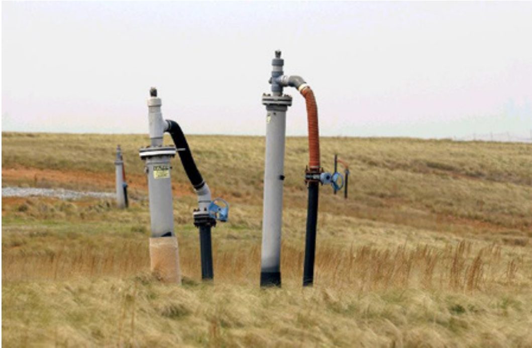
Figure 13.8 External Housing of a Landfill Gas Well
