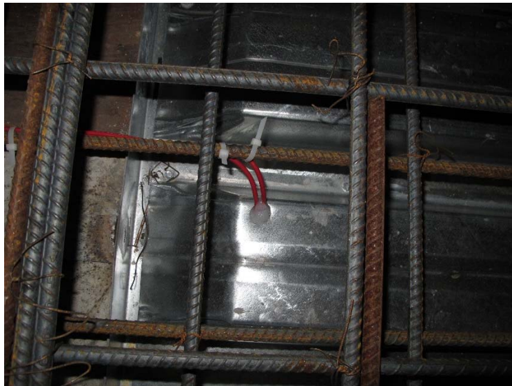
Figure 3.32: Wires passing through the deck
