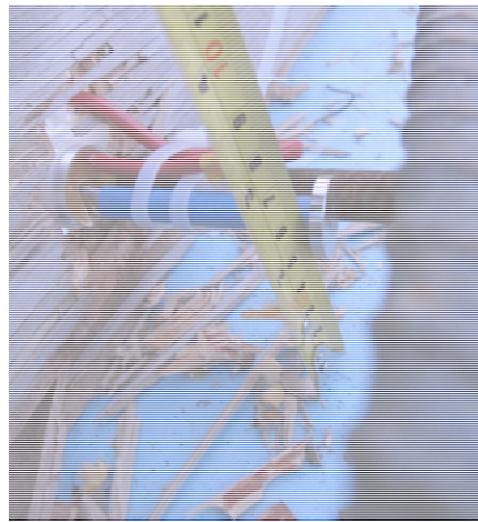
Figure 3.45: Gage through the Crack Former
