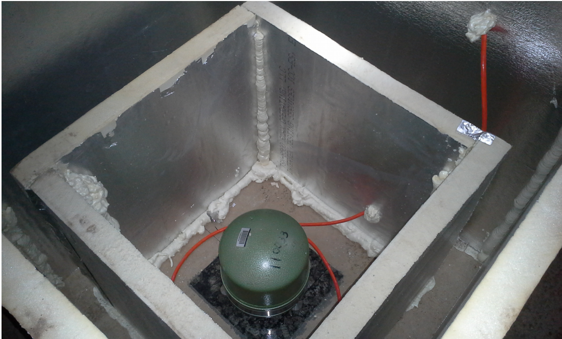
Figure 6.8: An example of the enclosure used for seismometers underground. This was taken at the B4850 station.
