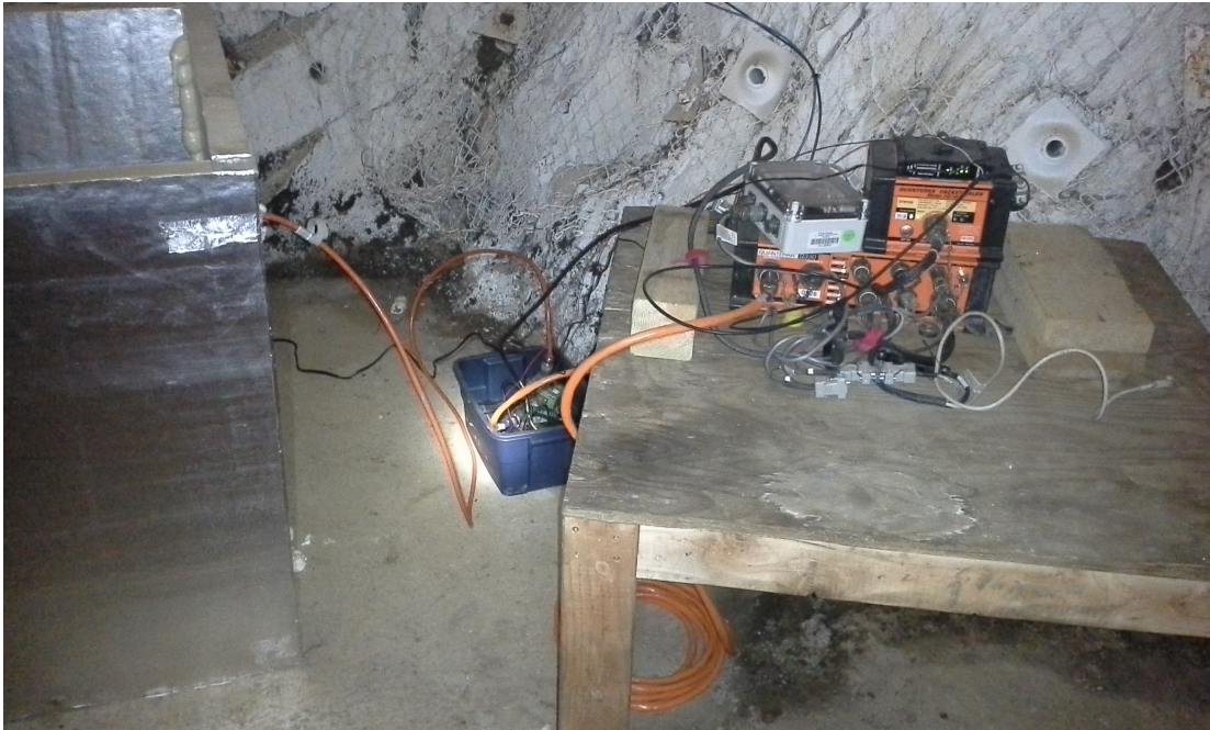
Figure 6.9: A full underground station set-up, with plastic tubs removed to show the electronics. This was taken at the B4850 station.
