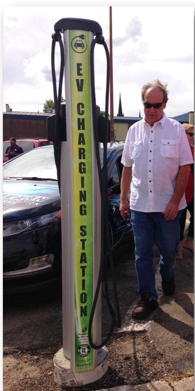
Charging Station, Austin Utilities
