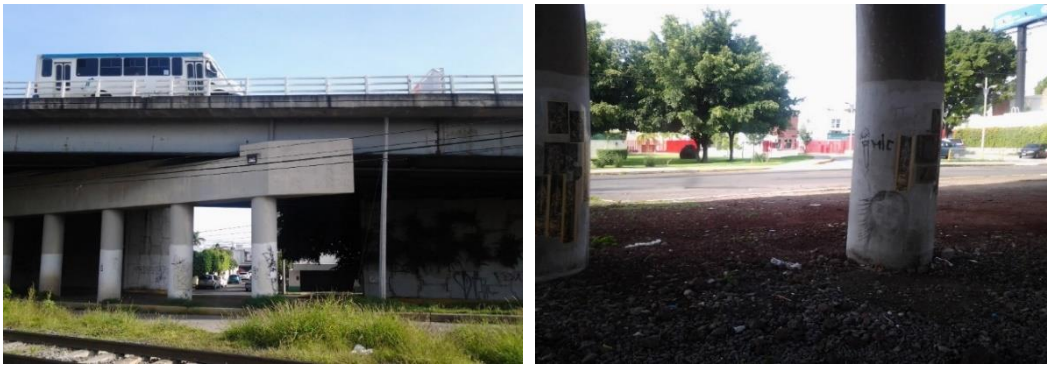
Illustration 25: The railroad tracks through the bridge. Photo taken during the summer of 2014.
