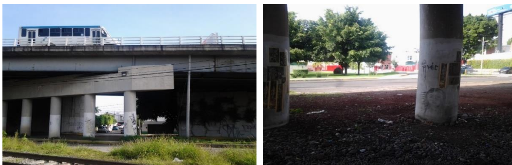
Illustration 3: The railroad tracks through the bridge. Photo taken during the summer of 2014.
