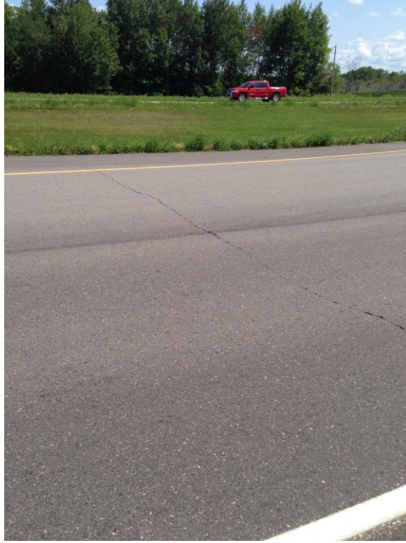
TH 10-typical crack configuration
