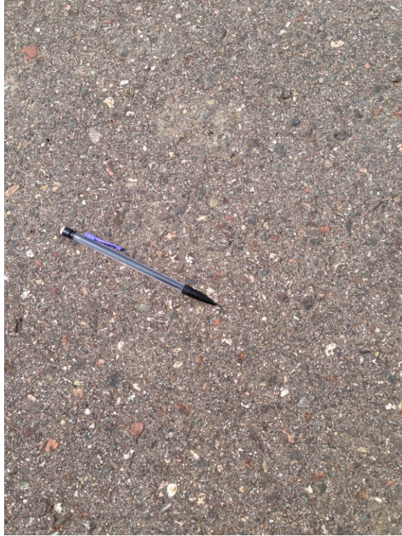
CSAH 10 poor performer-surface profile
