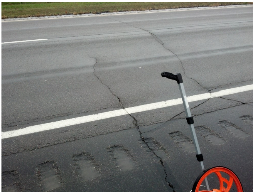
TH 10 good performer-typical crack configuration
