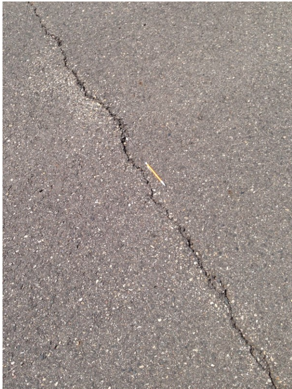
TH 220-typical crack profile
