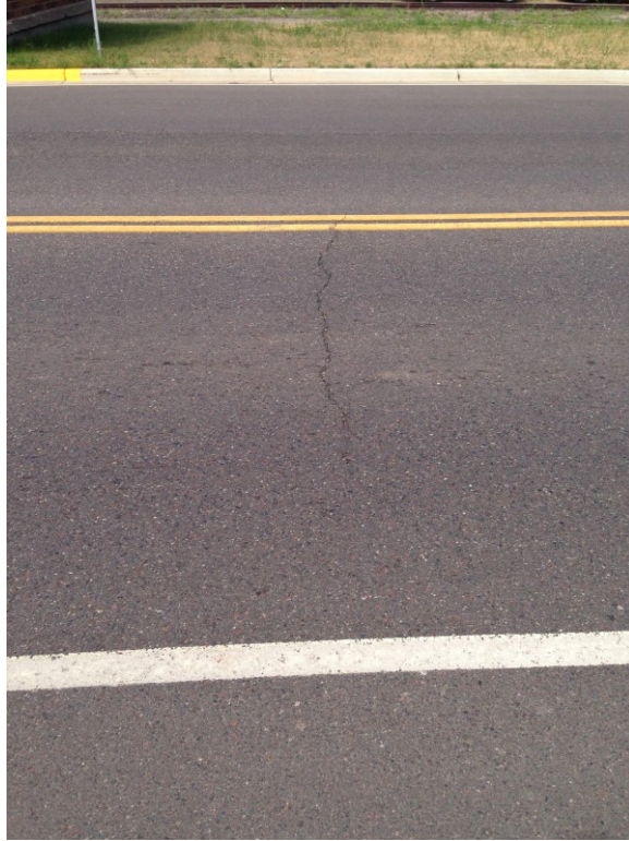
CSAH 30-typical crack profile
