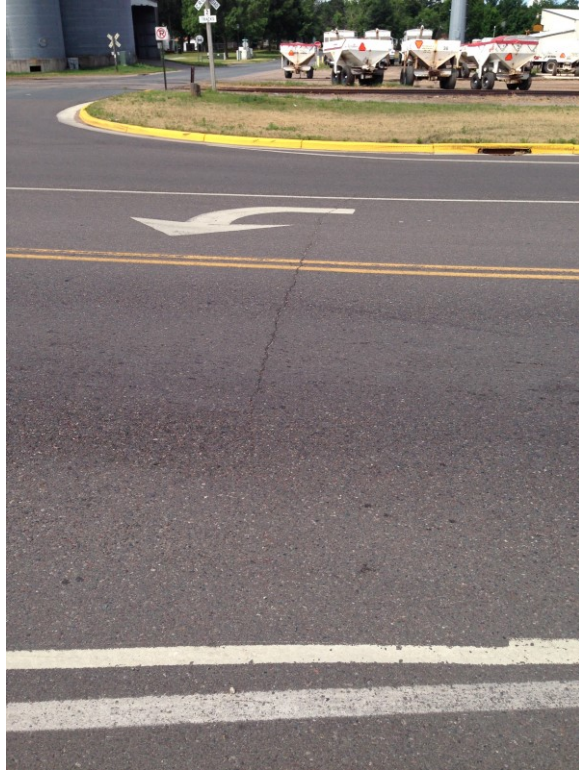
CSAH 30-typical crack configuration
