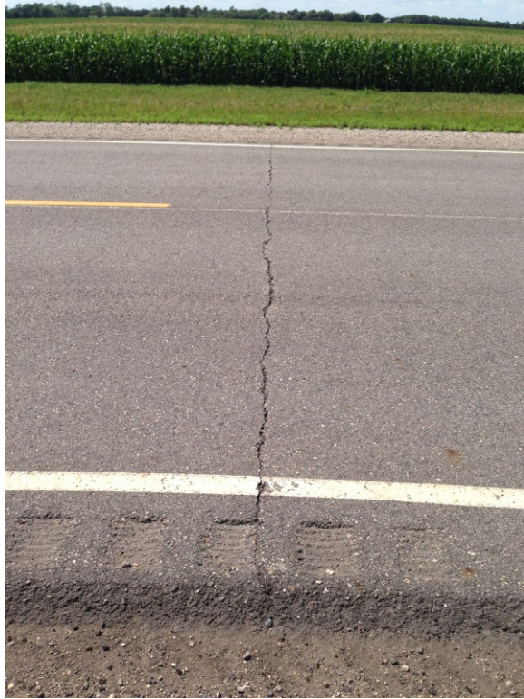
TH 220-typical crack configuration
