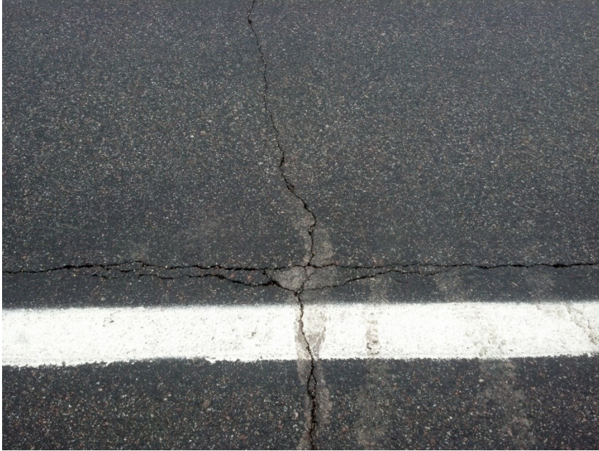
TH 10 good performer-typical crack profile and surface profile
