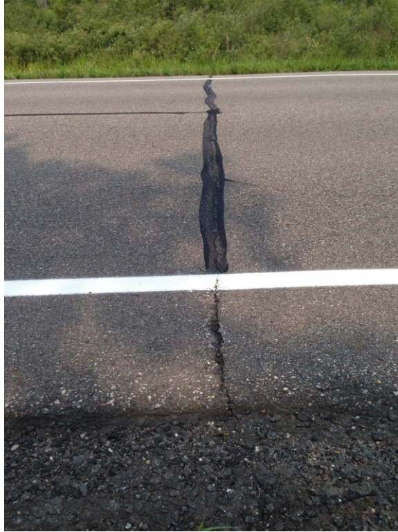
TH 6-typical crack profile
