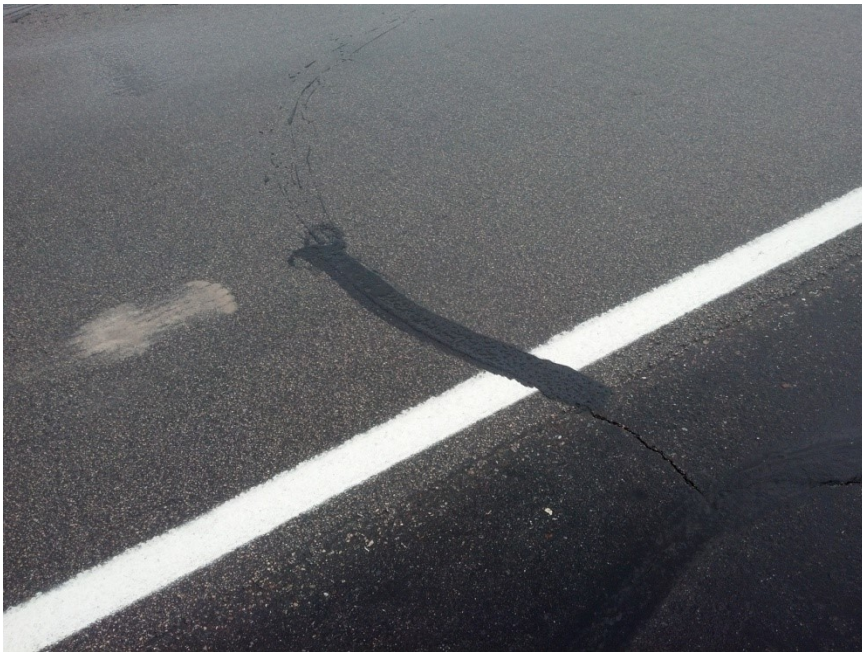
TH 10 poor performer-typical crack profile and surface profile
