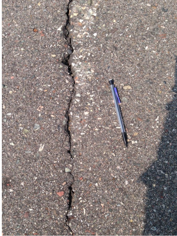
CSAH 10 good performer-typical crack profile
