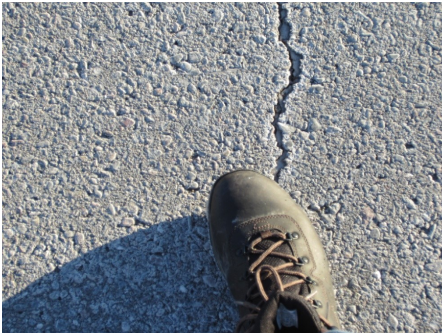
TH 210-typical crack profile
