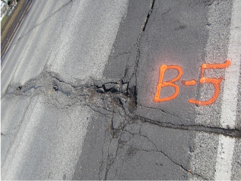
Figure 3.29 Pothole B-5 before Milling.
