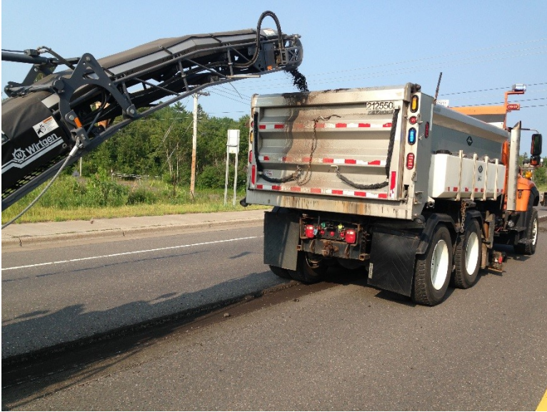
Figure B10: Milled Material is placed in a Truck to be Hauled Away.
