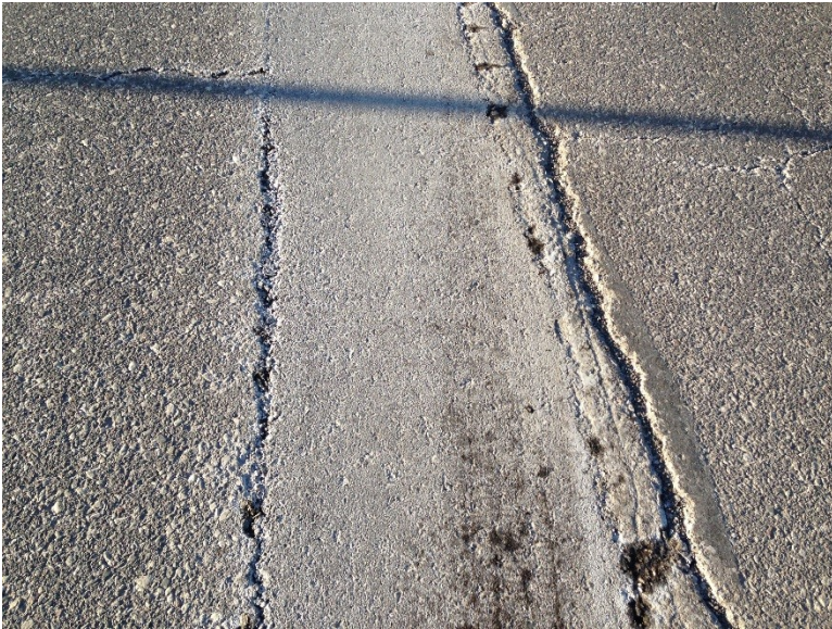
Figure 3.85 Close View of Distresses on Pothole E-5 (119 Days after Installation).
