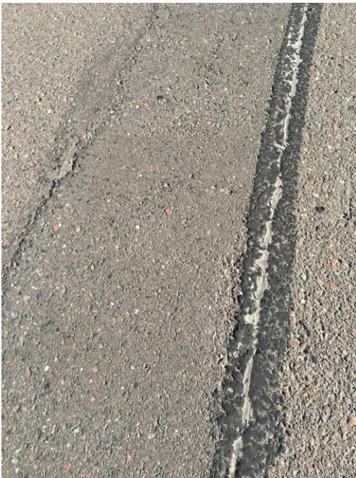
Figure 3.70 Pothole D-2 (426 Days after Patching).
