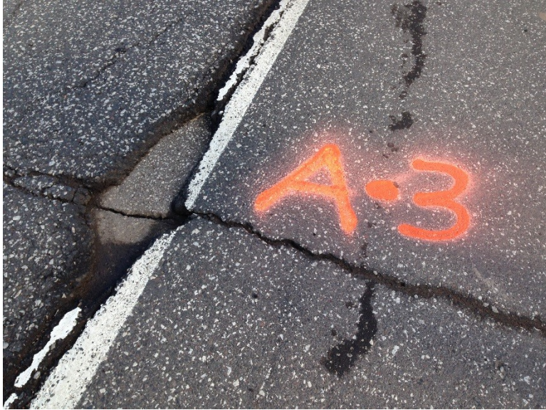
Figure 3.3 Pothole A-3 prior to Patching (After Cleaning).
