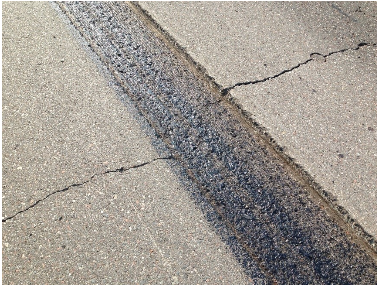
Figure 3.58 Milled Trench with Transverse Crack (Pothole D-3 Location).
