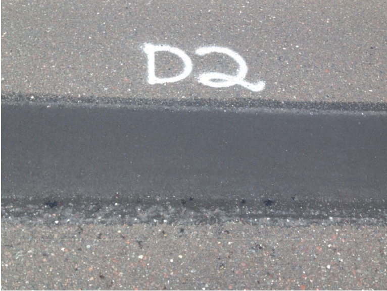
Figure 3.64 Pothole D-2 (35 Days after Patching).
