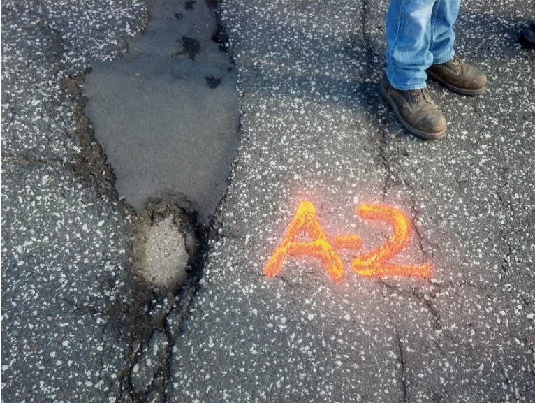
Figure 3.2 Pothole A-2 prior to Patching (After Cleaning).
