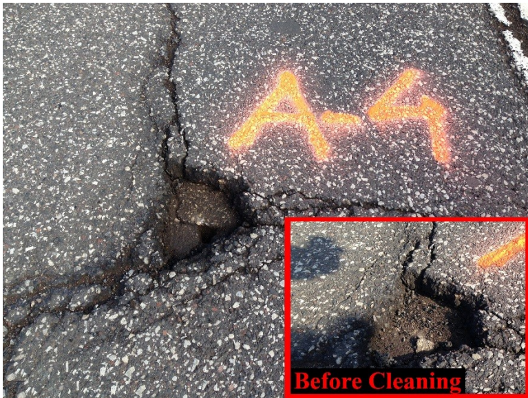
Figure 3.4 Pothole A-4 prior to Patching (Before and After Cleaning).
