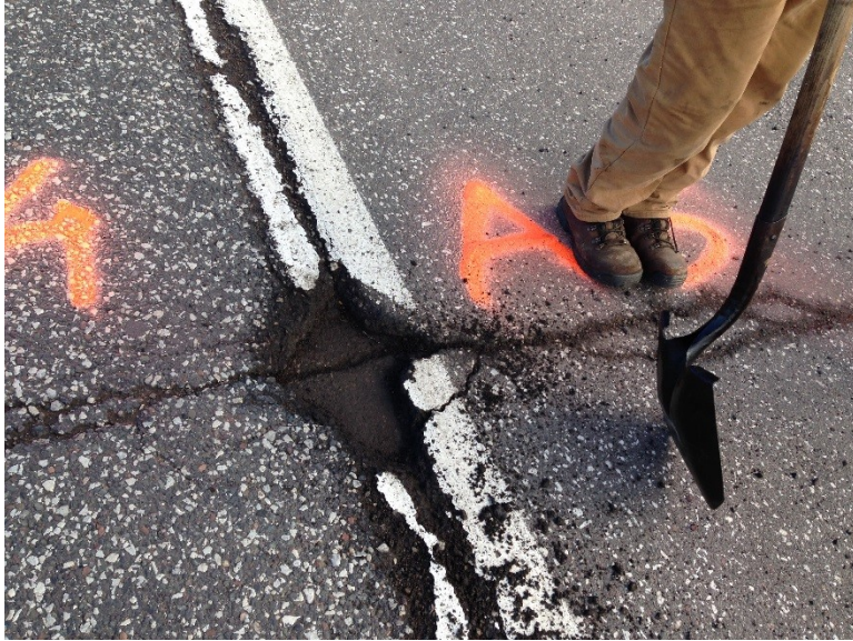
Figure 3.5 Pothole A-5 prior to Patching (After Cleaning).
