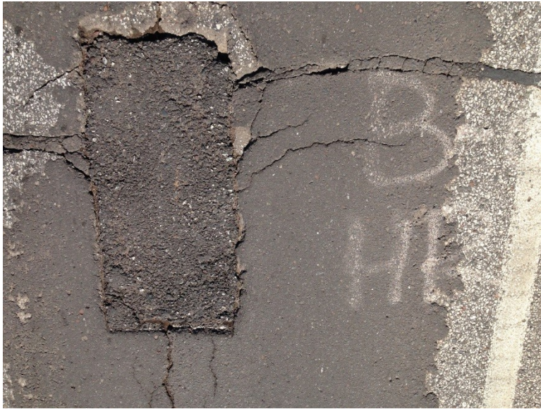
Figure 3.47 Pothole B-6 (146 Days after Patching).
