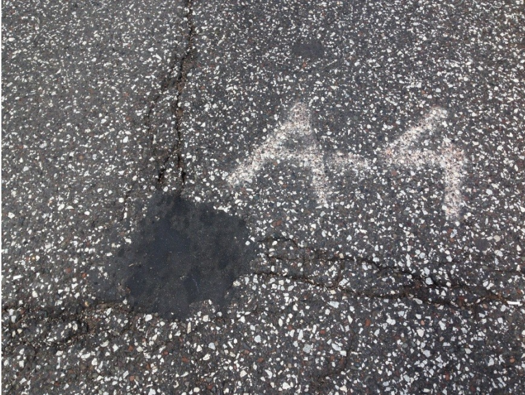
Figure 3.16 Pothole A-4 (149 Days after Patching).
