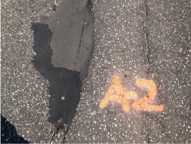
Figure 3.11 Pothole A-2 (3 Days after Patching).
