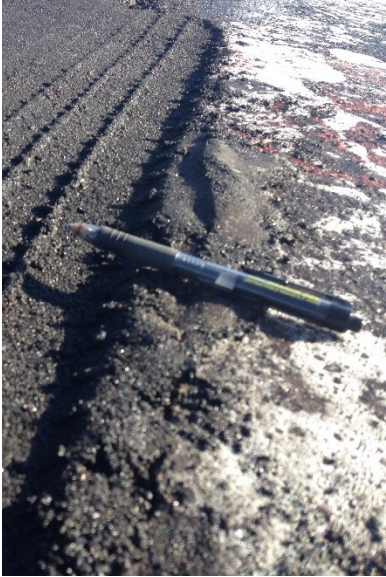
Figure 3.38 Settlement (Dishing) of Pothole B-2 an Hour after Compaction.
