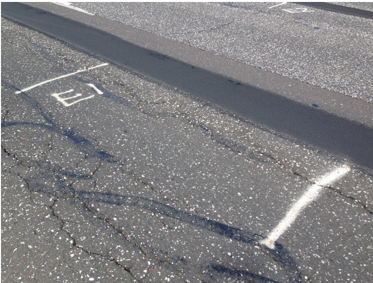
Figure 3.81 Patch E-1 Parallel to Existing Distresses (28 Days after Patching).
