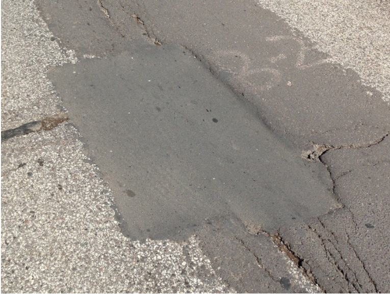
Figure 3.40 Pothole B-5 (146 Days after Patching).
