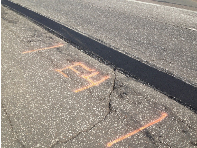
Figure 3.75 Pothole E-4 with Transverse Crack.
