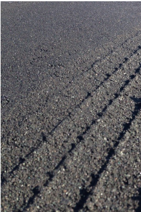
Figure 3.33 Settlement (Dishing) of Pothole B-2 an Hour after Compaction.
