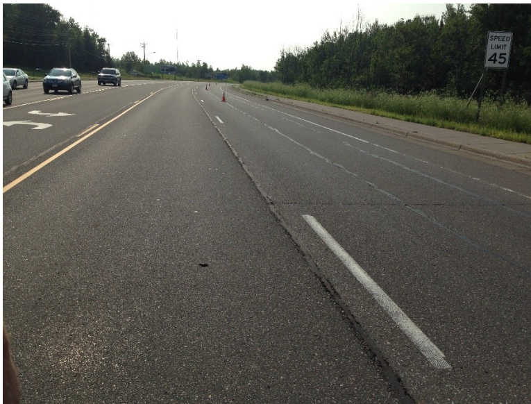
Figure 3.55 Longitudinal Crack along Trinity Road.
