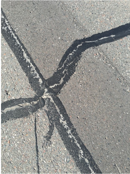
Figure 3.71 Pothole D-3 (446 Days after Installation) with Crack Running Through Patch.
