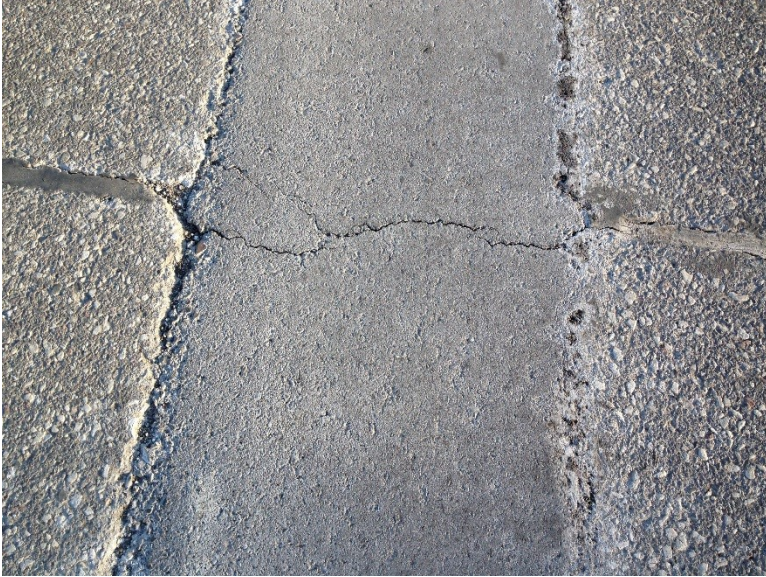
Figure 3.82 Cracking of Pothole E-3 (119 Days after Installation).
