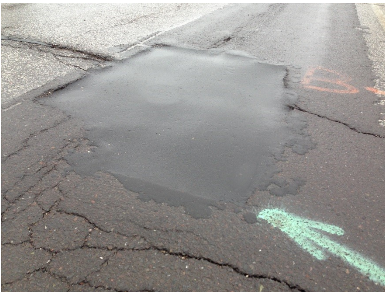
Figure 3.41 Water Accumulation in Dished Areas of Patch B-3 (18 Days after Patching).
