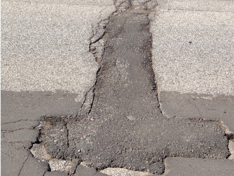
Figure 3.44 Pothole B-5 (146 Days after Patching).
