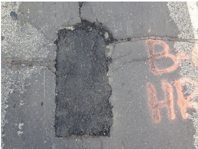
Figure 3.46 Pothole B-6 (3 Days after Patching).
