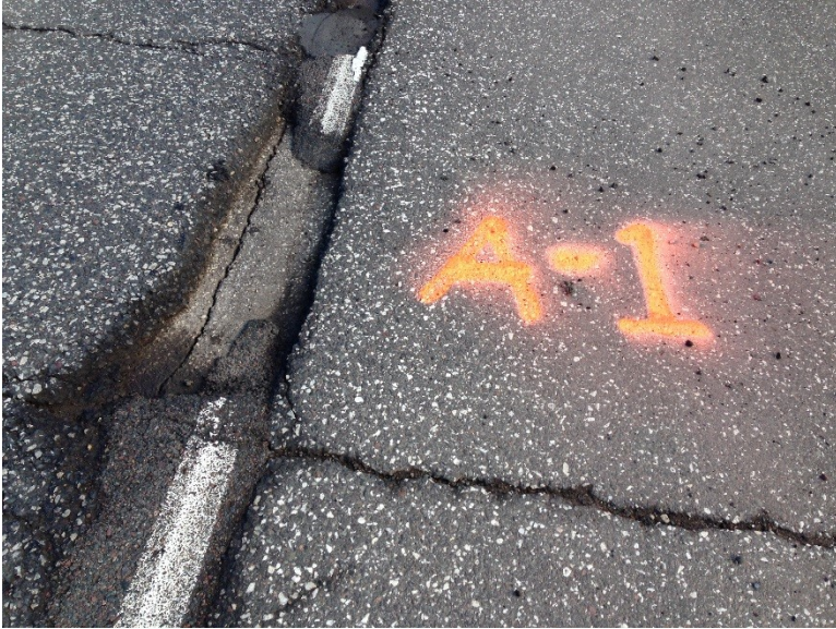
Figure 3.1 Pothole A-1 prior to Patching (After Cleaning).
