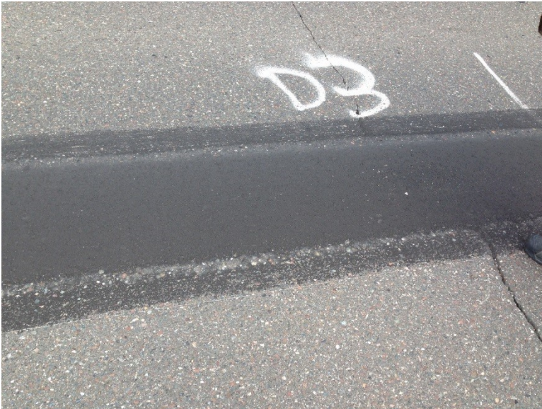
Figure 3.65 Pothole D-3 (35 Days after Patching).
