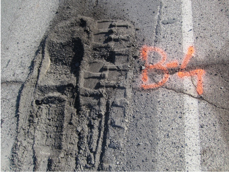
Figure 3.28 Pothole B-4 with Milling Debris Still in Place.
