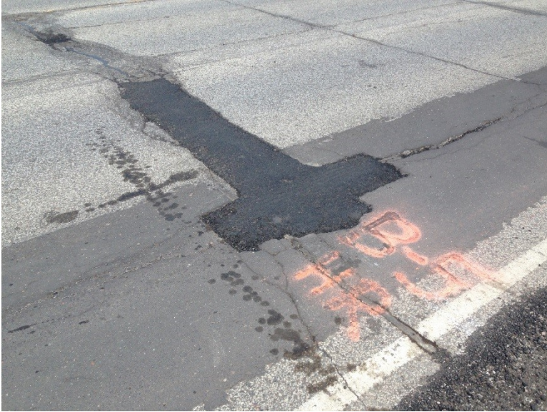
Figure 3.43 Pothole B-5 (3 Days after Patching).
