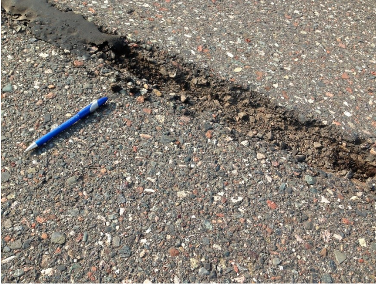
Figure 3.56 Section of Longitudinal Crack with Sealer Missing.
