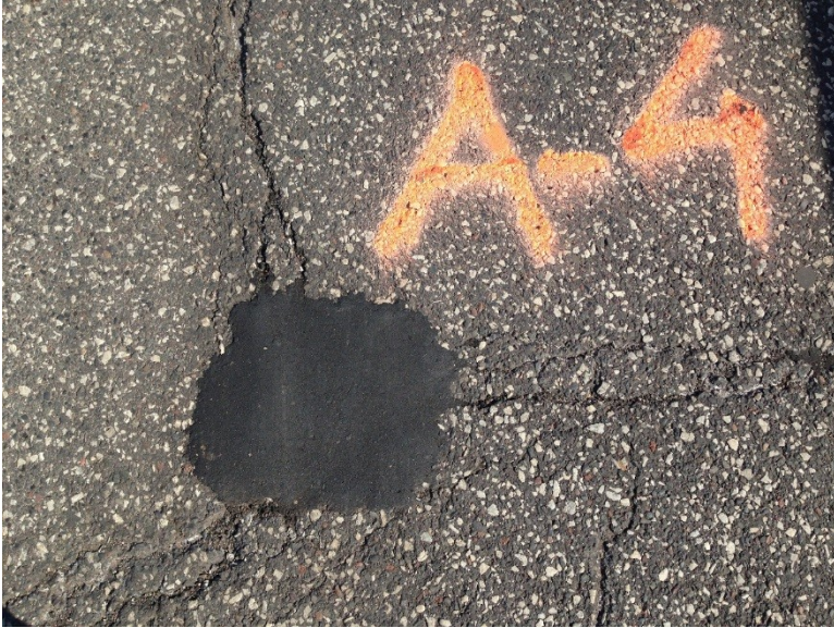
Figure 3.15 Pothole A-4 (3 Days after Patching).
