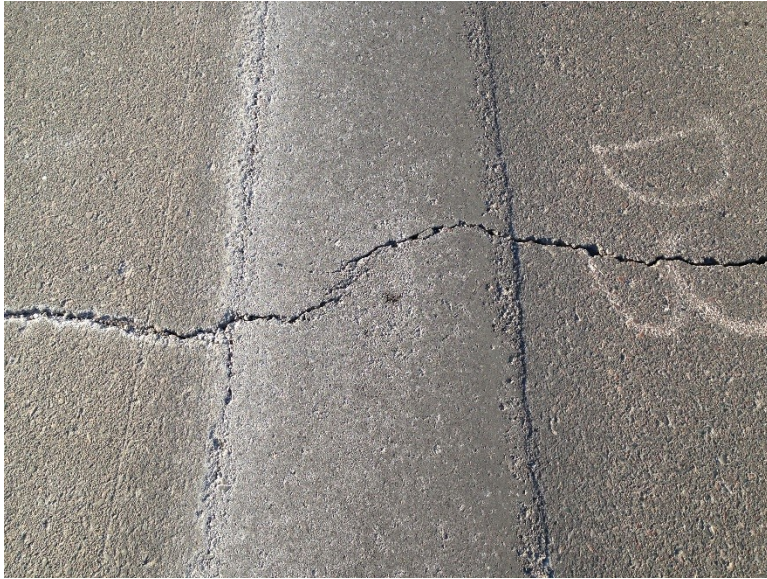
Figure 3.68 Pothole D-3 (126 Days after Installation) with Crack Running Through Patch.
