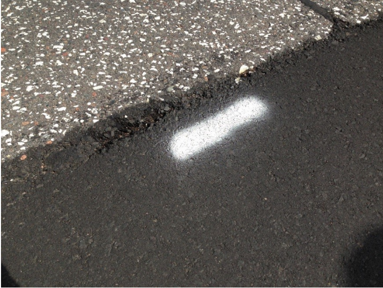
Figure 3.80 Poorly Compacted Interface (28 Days after Patching).
