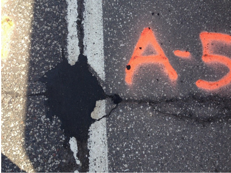
Figure 3.17 Pothole A-5 (3 Days after Patching).
