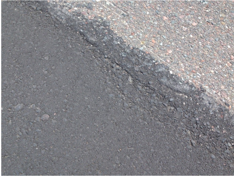
Figure 3.66 Patch Interface (35 Days after Patching).
