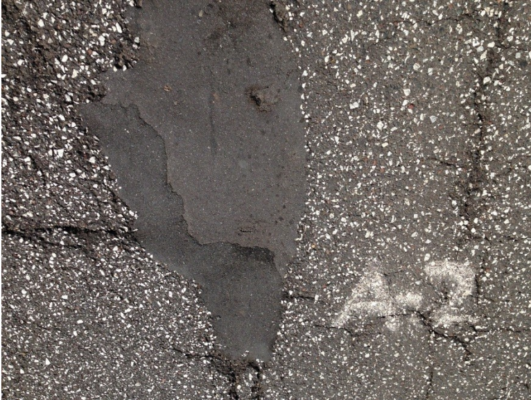
Figure 3.12 Pothole A-2 (149 Days after Patching).
