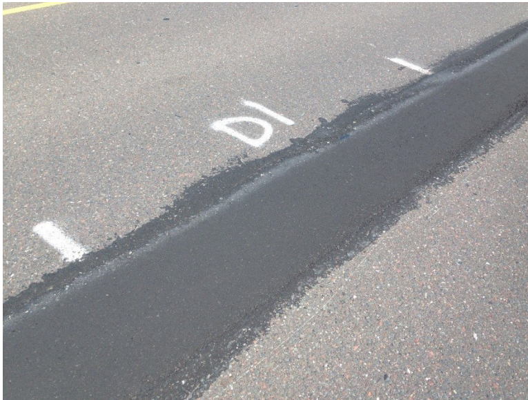
Figure 3.63 Pothole D-1 (35 Days after Patching).
