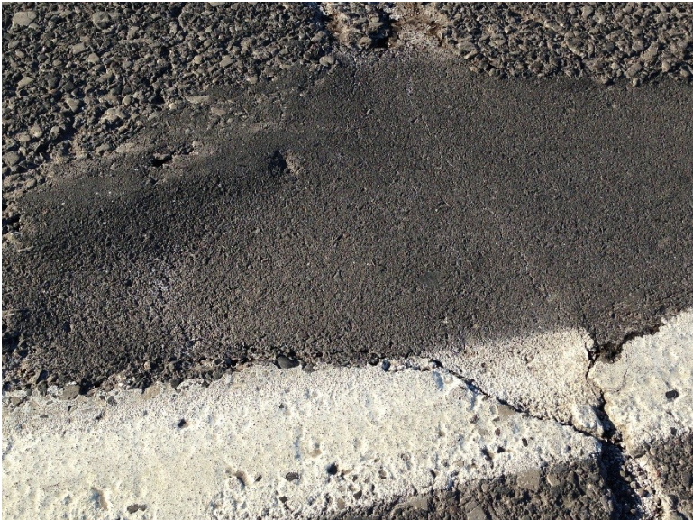
Figure 3.20 Pothole A-5 (240 Days after Installation).
