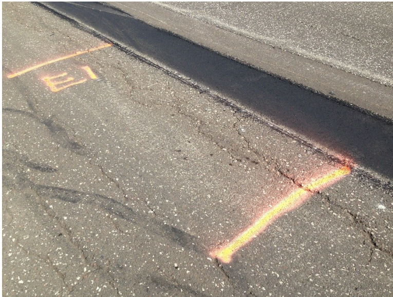
Figure 3.72 Pothole E-1 with Parallel Longitudinal Cracking.
