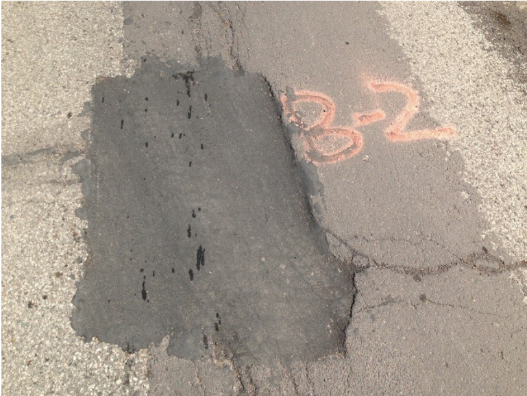
Figure 3.39 Pothole B-2 (3 Days after Patching).
