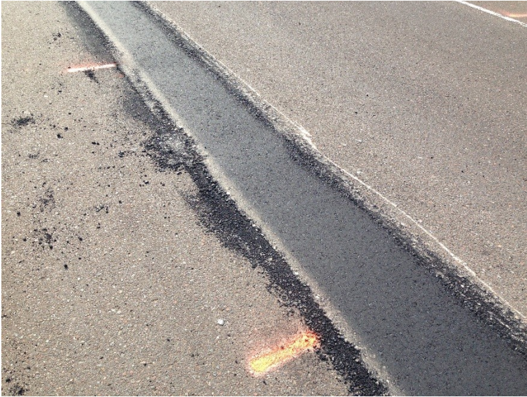
Figure 3.59 Pothole D-1 after Compaction (Excess Fill Material on Roadway).
