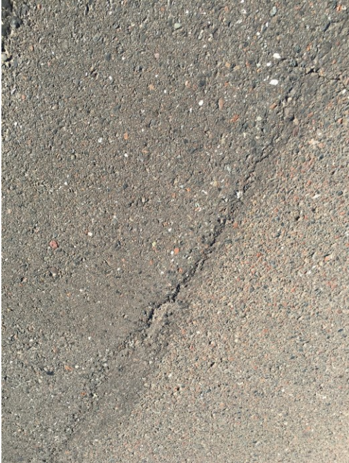
Figure 3.69 Pothole D-1 (446 Days after Installation).
