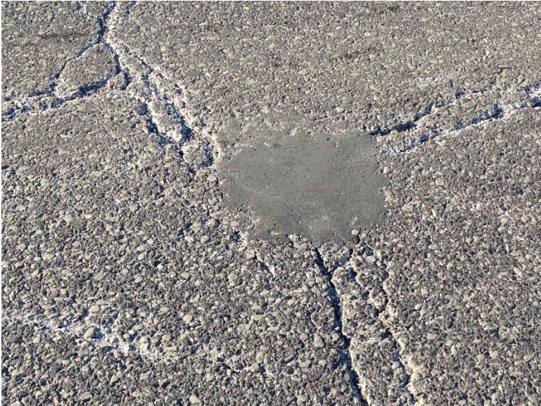
Figure 3.19 Pothole A-4 (240 days after installation) with Snow Plow Abrasion.
