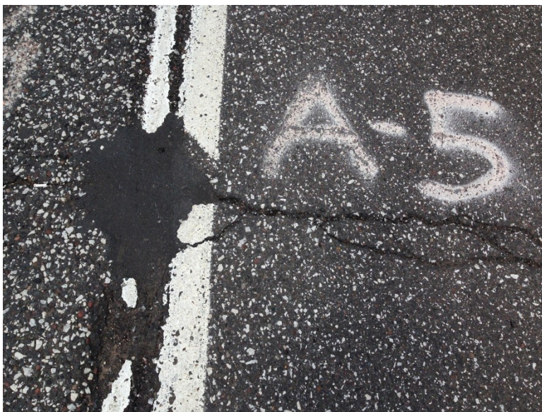
Figure 3.18 Pothole A-5 (92 Days after Patching).
