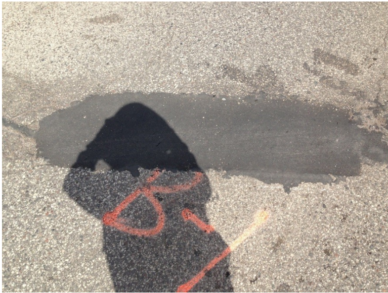
Figure 3.37 Pothole B-1 (3 Days after Patching).
