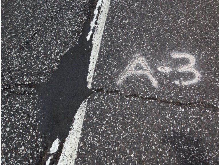
Figure 3.13 Pothole A-3 (149 Days after Patching).
