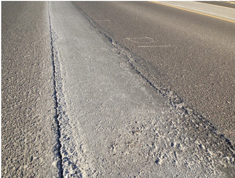
Figure 3.67 Pothole D-1 (126 Days after Installation) with Deterioration along the Patch Interface.
