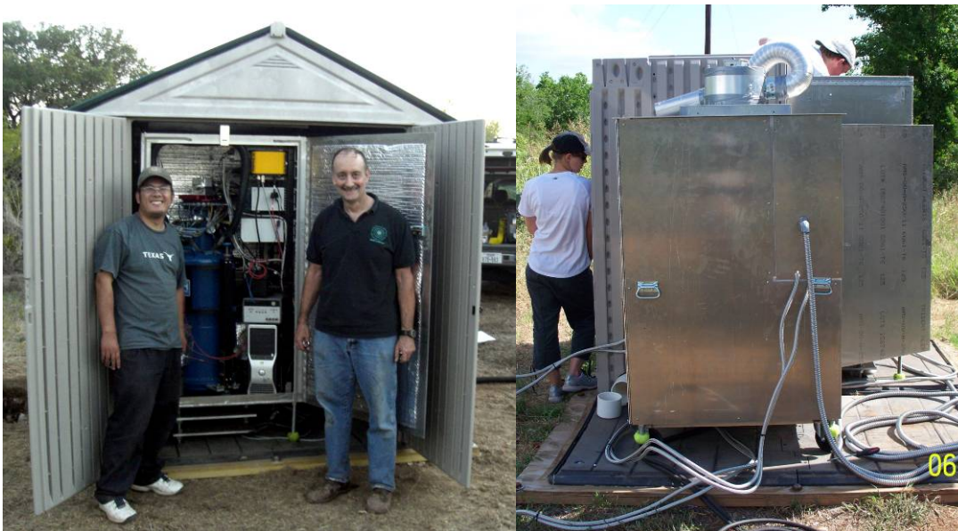
Figure 2.17: Pictures taken at Green Emerald Terrace when gravimeter installation completed. The left panel shows gravimeter shed, shed door and enclosure door opened. Right panel shows refrigerator shed.
