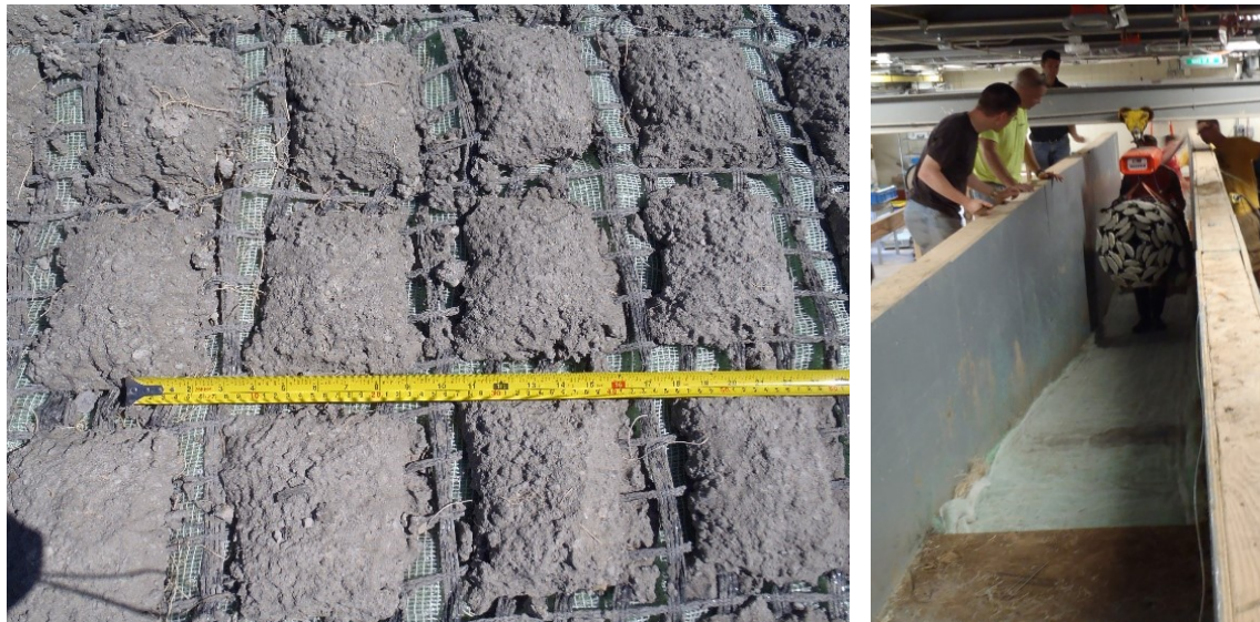
Figure 3.14. Photo on the left shows the concrete blocks and flexible geogrid underlain by the turf reinforcement mat. In the photo on the right, the turf reinforcement mat is overlaying the soil and the concrete blocks and flexible geogrid is being hoisted into place.
