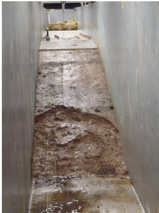
Figure 4.57. Looking upstream from run-out area. Stabilization material removed showing the extent of the erosion starting at the toe of the slope and working up towards the shoulder.
