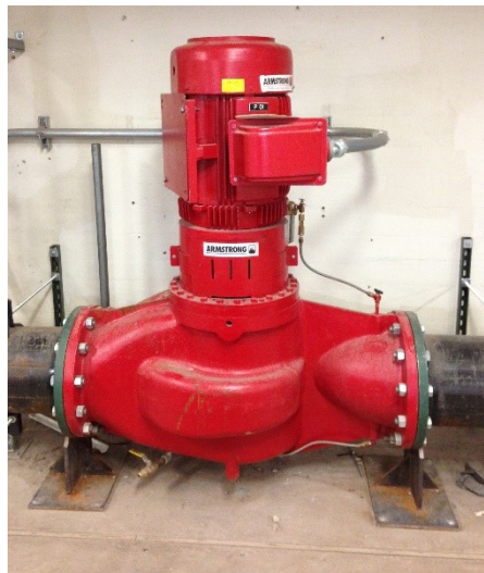
Figure 3.4. Pump #1 on the model floor.
