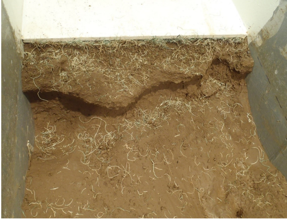
Figure 4.48. Looking upstream at shoulder and slope after stabilization material was removed. Note the remaining soil that was not undermined but close to it after 6 hours of run time.
