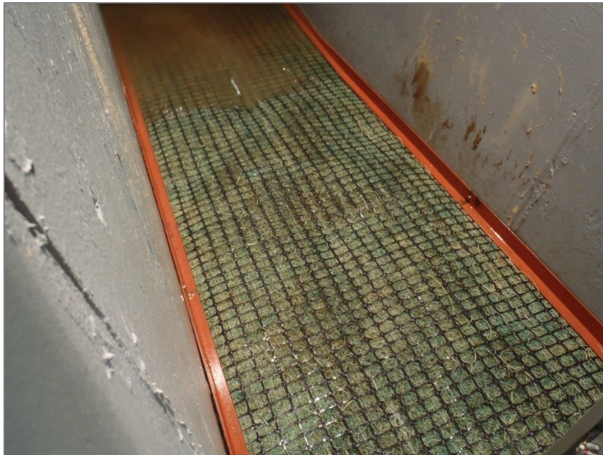
Figure 4.30. Image of early sign of erosion as a depression 75% of the way down slope caused water to separate from bed. Image is looking downstream near toe of slope with tail-water still draining.
