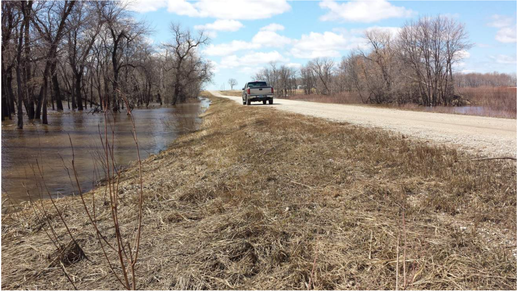
Location 5 looking west at the downstream shoulder, post-flooding condition
