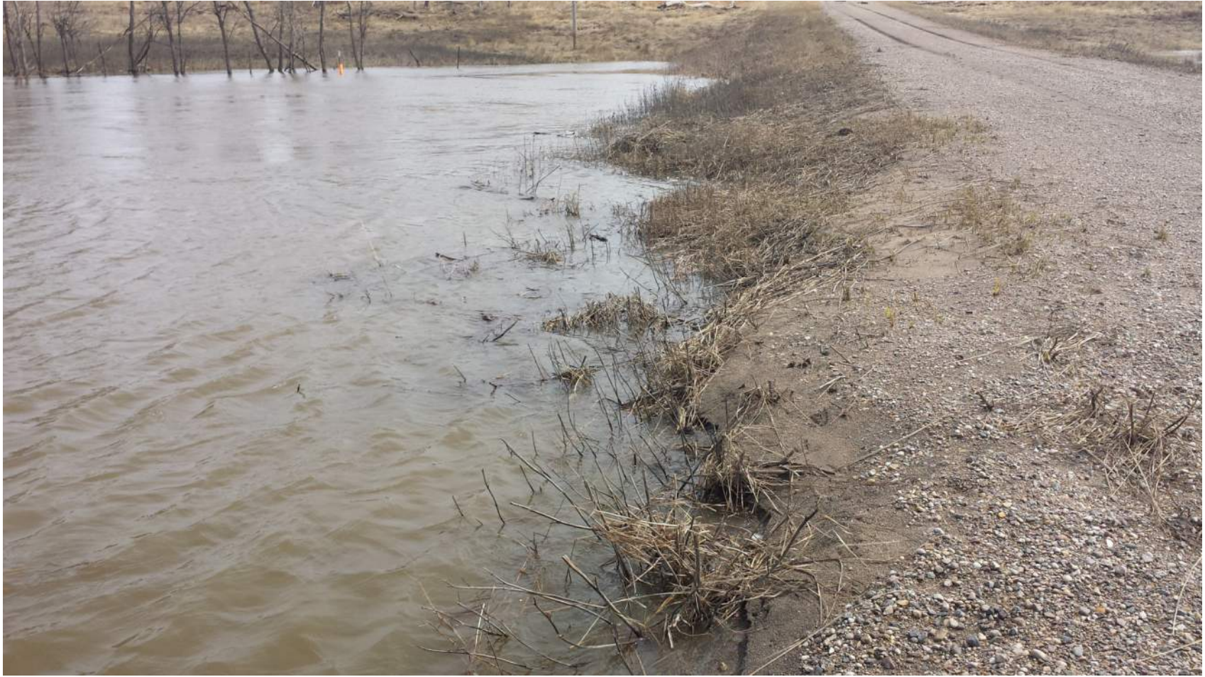
Location 4 looking east at minor erosion and deposition on the downstream shoulder, post-flooding condition
