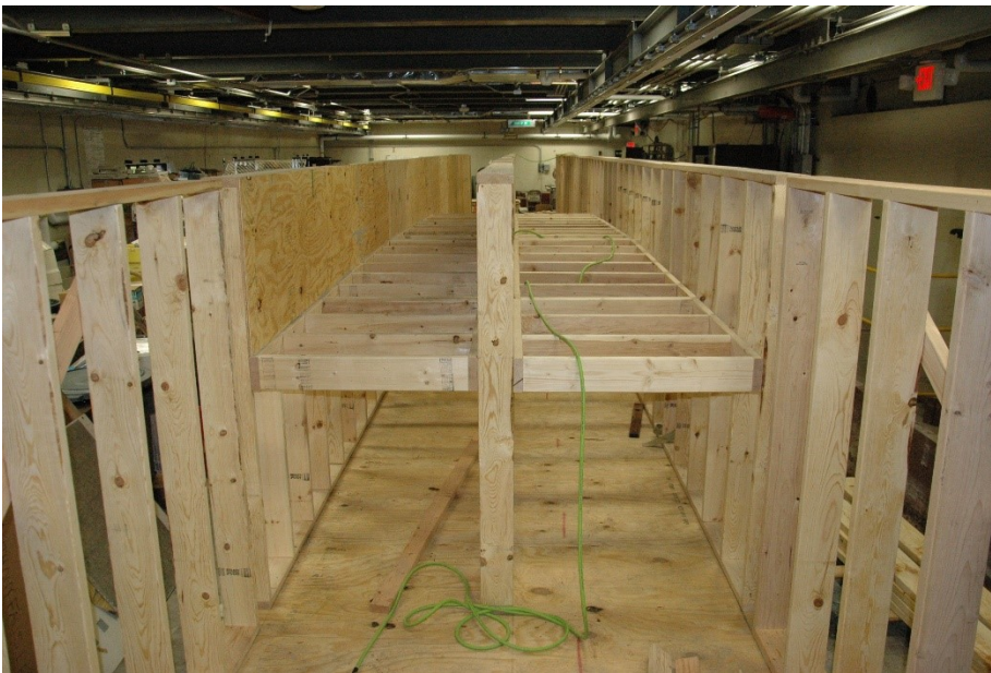
Figure 3.2. Flume during construction. Looking downstream from the headbox. The 6H:1V slope is to the left of the center wall, and the 4H:1V slope is to the right of the center wall.
