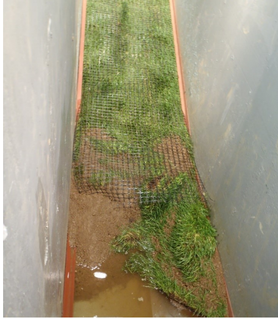
Figure 4.56. Looking upstream at toe of slope. Erosion beginning at toe of slope, undermining sod and washing some pieces away. Erosion working up the slope from run-out area.
