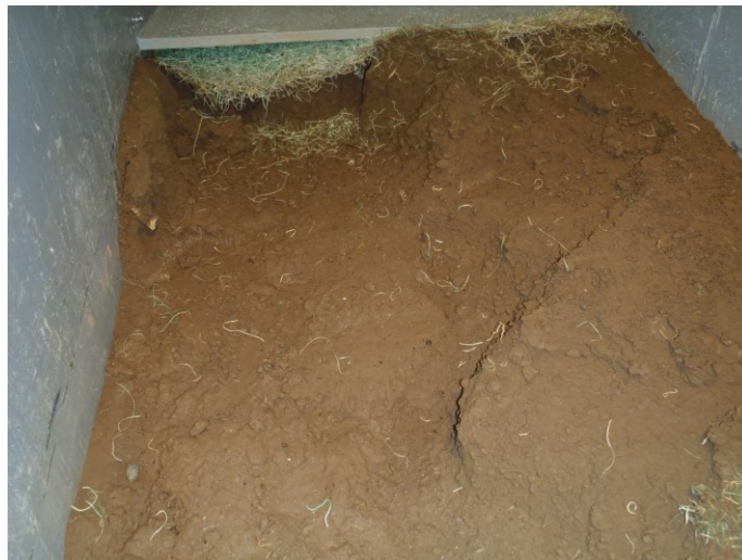
Figure 4.23. Slope with the shoulder at the top of the photo after ECB was removed post-testing. Note the undermining of shoulder and extensive erosion not seen with ECB still in place on previous photos.
