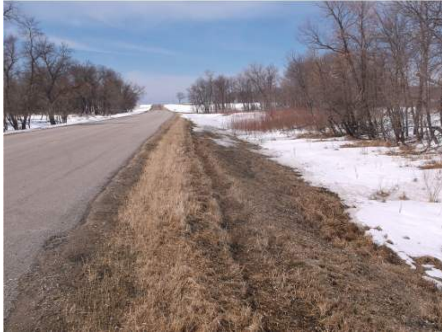
Existing Shoulder Conditions in Kittson County
