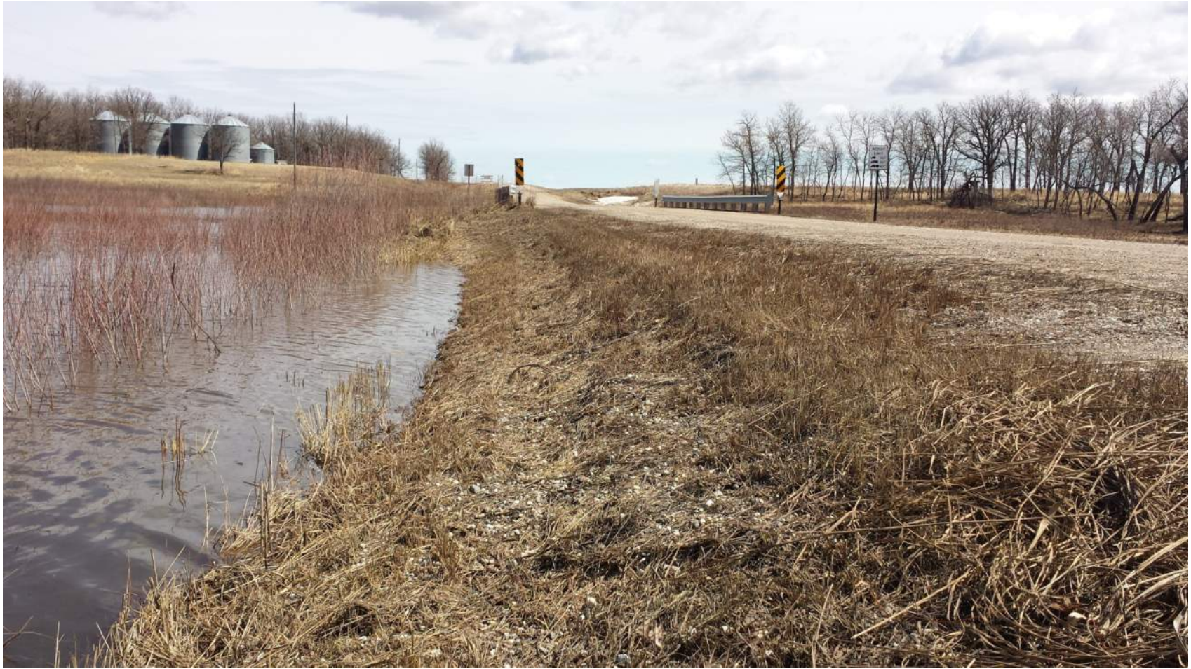
Location 5 Looking east at the upstream shoulder, post-flooding condition
