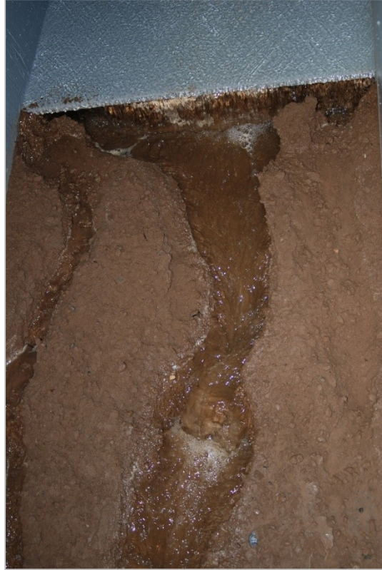
Figure 4.9. Channelized flow and separation from the edge of the shoulder forming trough at the transition.
