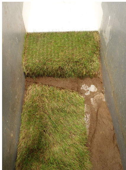
Figure 4.66. Looking upstream at shoulder to slope transition after the geogrid has been removed. Most of the transition is still intact while the areas where there was a seam between the rolled out pieces of sod allowed water to penetrate and erode the slope surface under the sod which was being partly held in place by the geogrid and landscaping staples.
