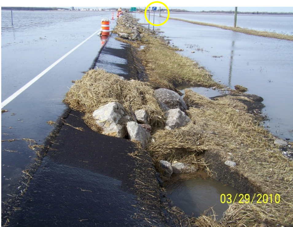
Figure 1.5. Same location, eight days later. Temporary stone fill dumped in some scour holes. Photo by JT Anderson, MnDOT.
