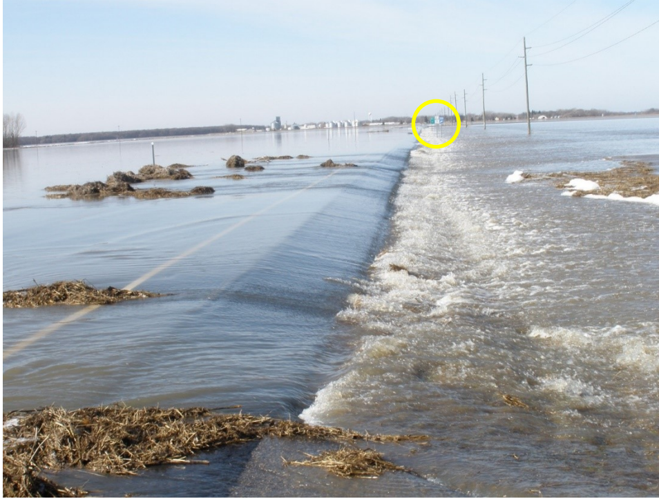
Figure 1.4. Overtopping event on MN TH1 near Oslo, Minnesota, March 21, 2010. “TH 1 at Jct 220 near Oslo 20100321”. Note road signs in yellow circle. Photo by JT Anderson, MnDOT
