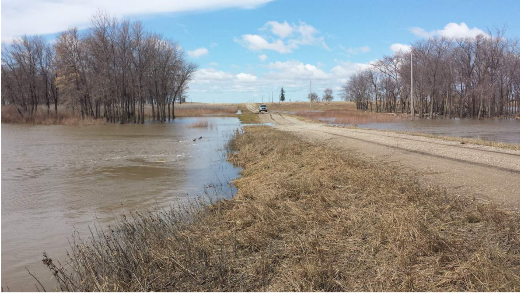
Location 4 Looking west at the upstream shoulder, post-flooding condition
