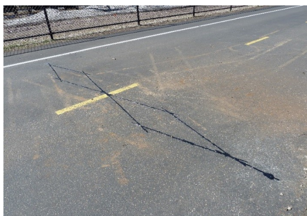
Figure 17: Sealed In-Pavement Inductive Loop
