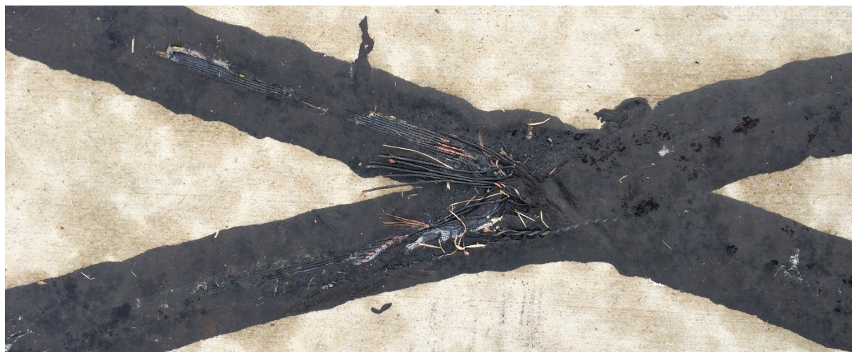
Figure 18: Inductive Loop on Top of Road Surface Worn and Frayed from Exposure and Road Maintenance
