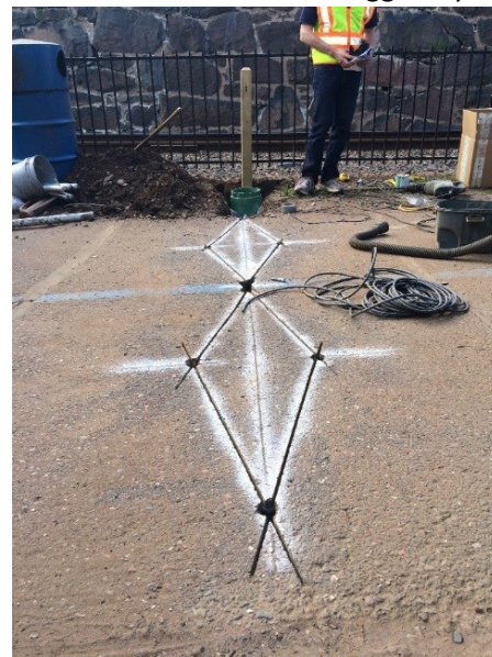
Figure 19: Inductive Loop and Infrared on Urban Multi-purpose Path
