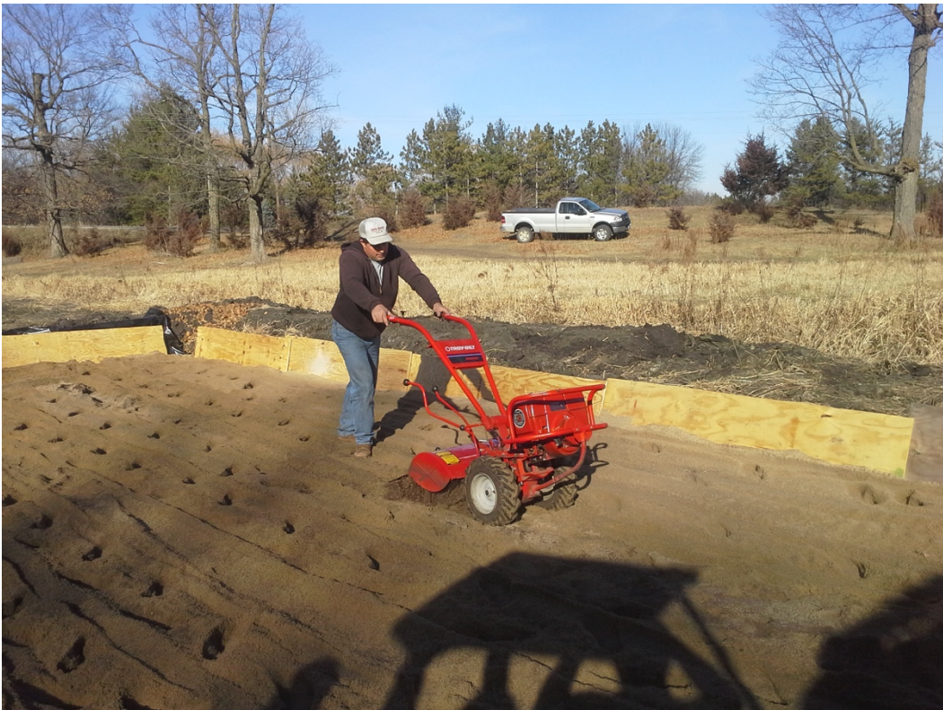
Figure 34. Construction: iron aggregate being mixed with sand by rototiller. Note: Sheet plywood along perimeter to protect impermeable liner from rototiller blades.
