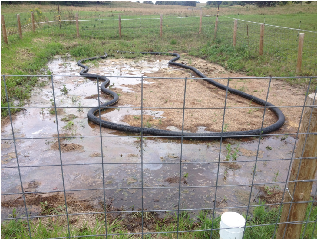
Figure 39. IESF after rainfall with standing water, vegetation, iron ochre, and algae. Black perforated distribution pipe shown on surface.
