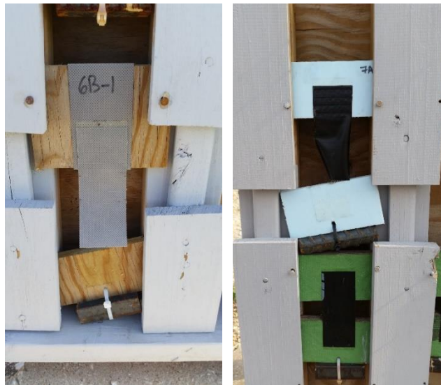
Figure 6.9: Combined Failure Mode.
