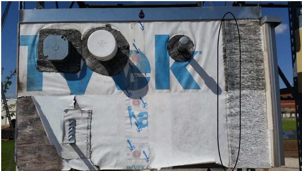
Figure 3.12: Fishmouthing Along the Flashing at The Window Flange Noticed in Specimen DRP1009-02.
