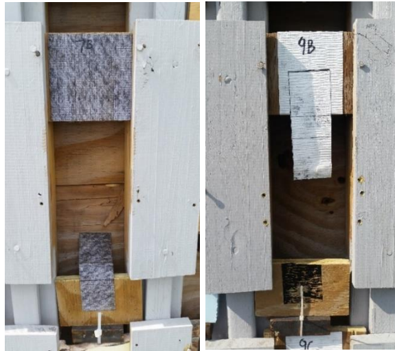
Figure 6.10: Failures Tape over Tape Scenario.
