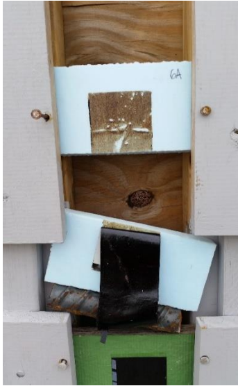
Figure 6.8: Bonding Incompatibility Between the Adhesive and the Substrate.
