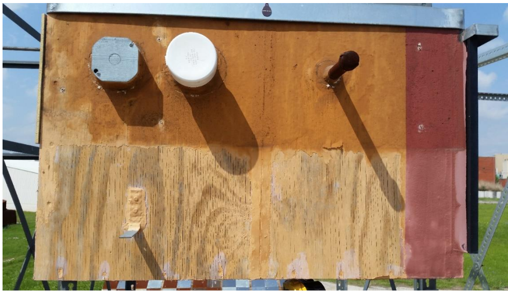
Figure 3.13: Specimen DRP1009-03 2.5 Years After Cladding Installed. The Exposed Part Has Washed Off.
