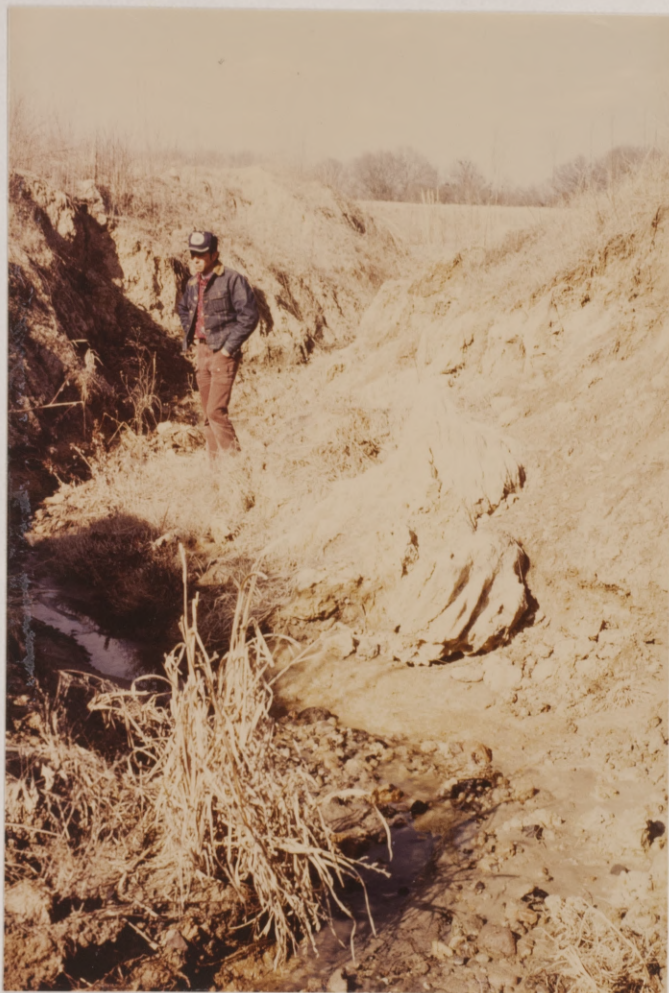
Figure 32. Deep gully at mine-site number Hp/Y-3-1, Hopkins County, Texas, 1980. The gully is cutting through 3 m of spoil material.
