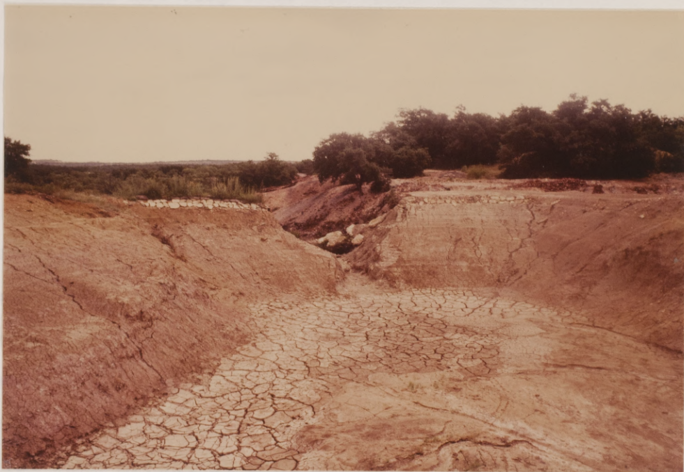
Figure 28. Failed earthen dam just below mine-site number Ea/CN-2-3, Eastland County, Texas, 1979.
