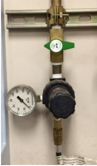
Figure 3.13: Compressed air valve and regulator for gas quenching.
