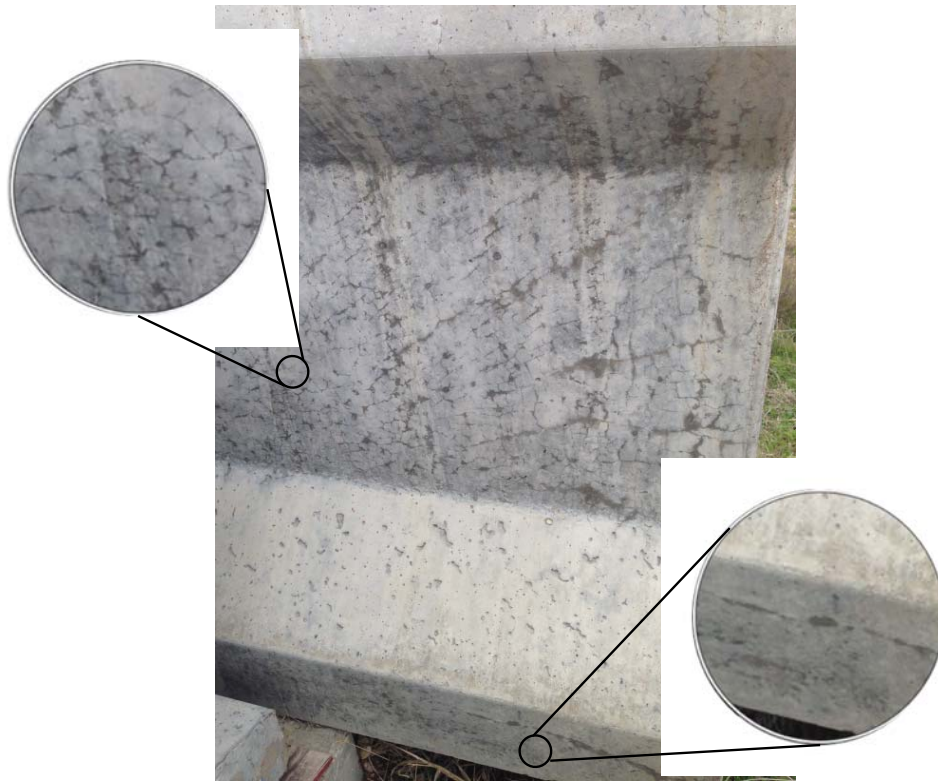
Figure 102: Girder located at PP-B: Concentration of Micro-cracking Focused on Girder Web
