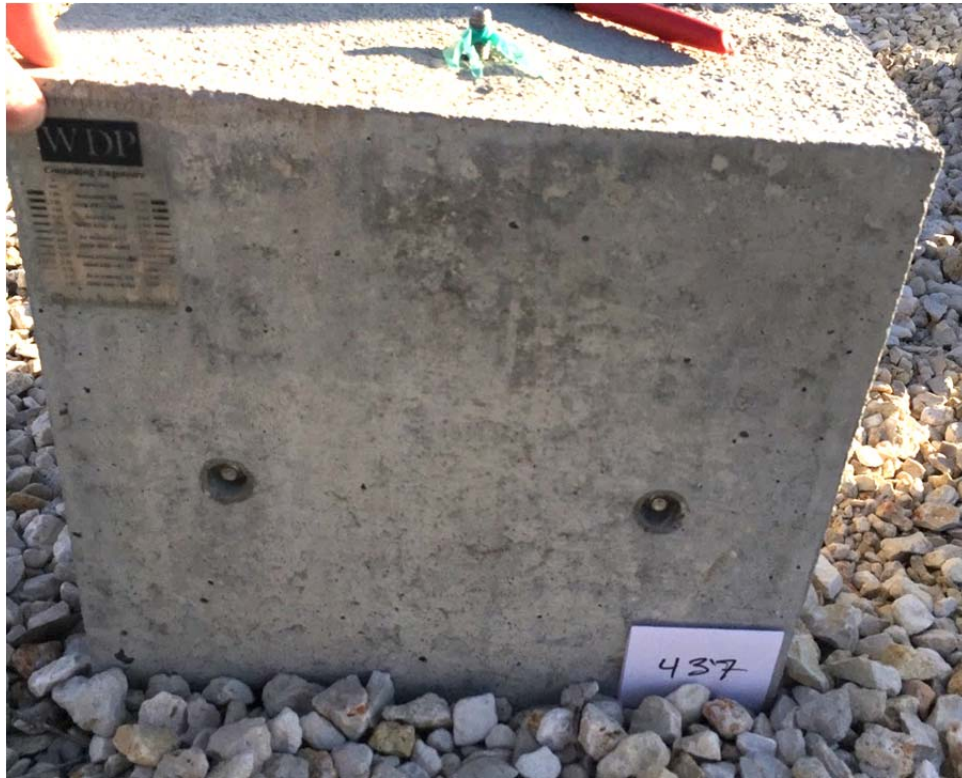
Figure 91: Example Crack Rating = 1
