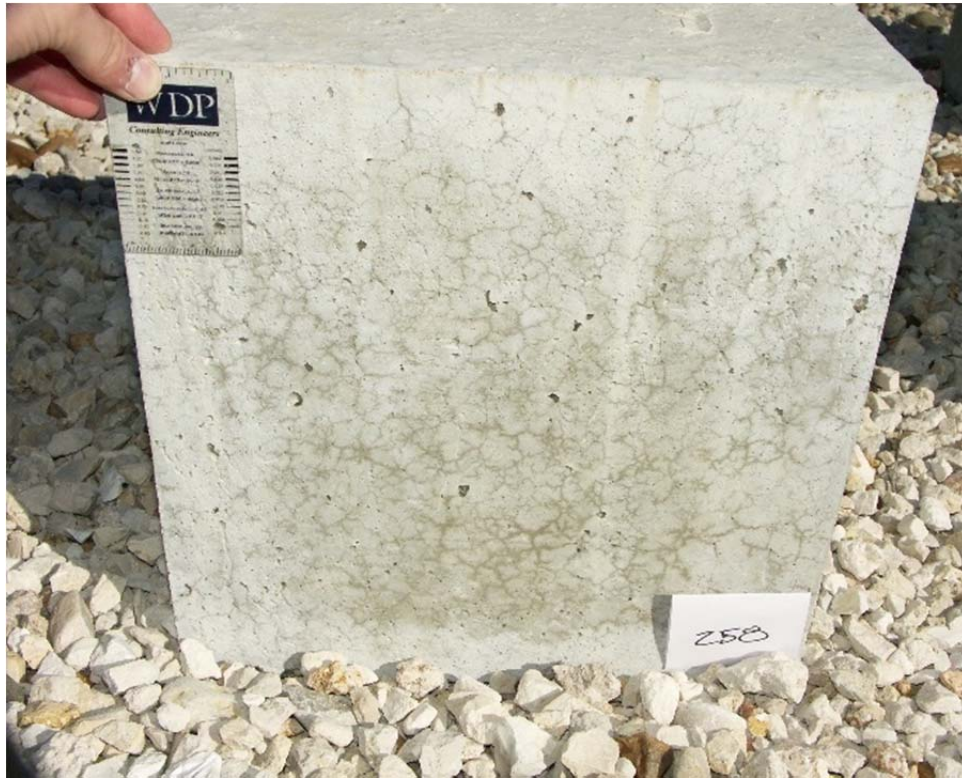
Figure 93: Example Crack Rating = 3
