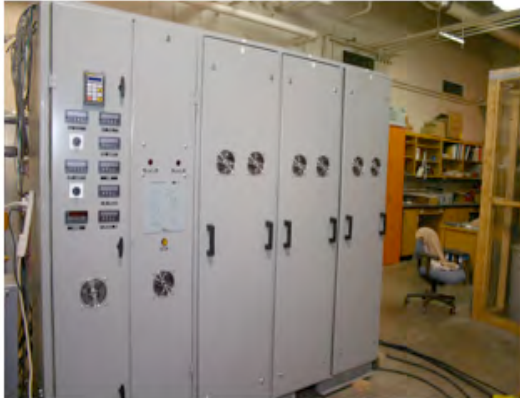
Figure 6. Photo of ARCP drive inverter for 2-MW flywheel motor-generator
