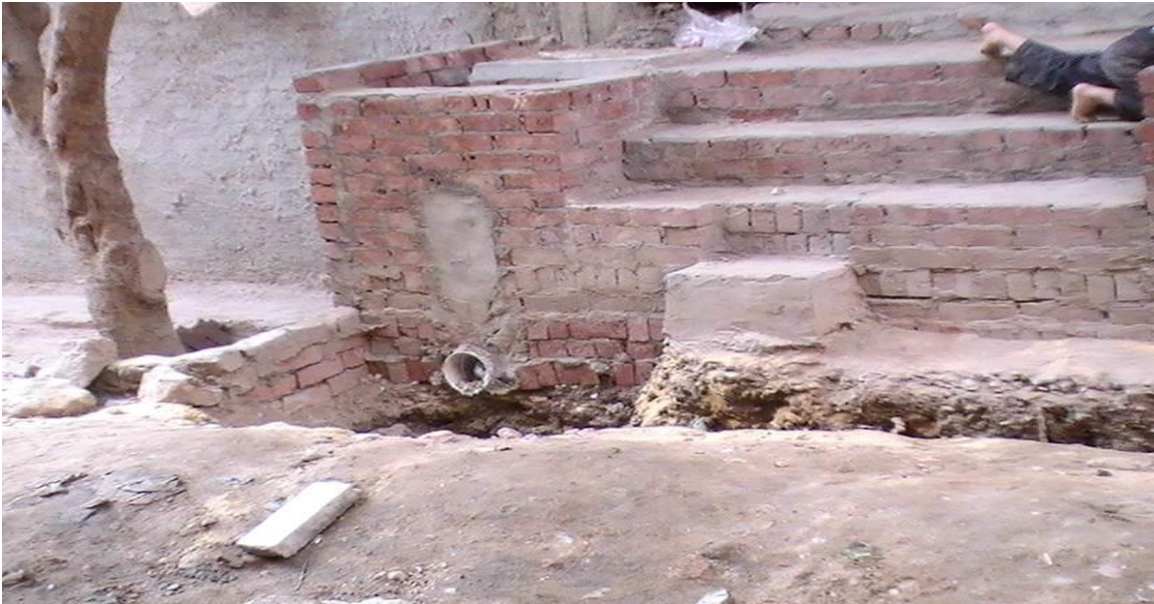
Figure 12: An outtake pipe made visible when trenches were being dug for the instillation of the new state run sewage system. Image by author, 2010.
