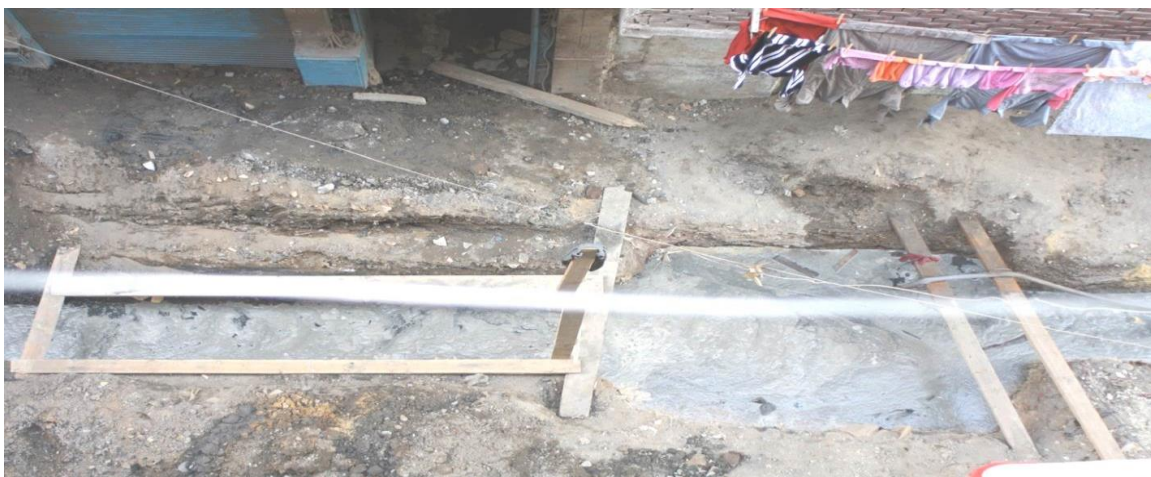
Figure 14: The view from Um Ameer’s balcony as the trench for the new septic system pipes filled up with water from a burst main. Image by author, 2010.
