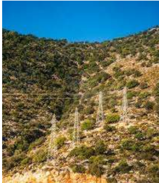
Figure 3. 2: Transmission line on a hill
