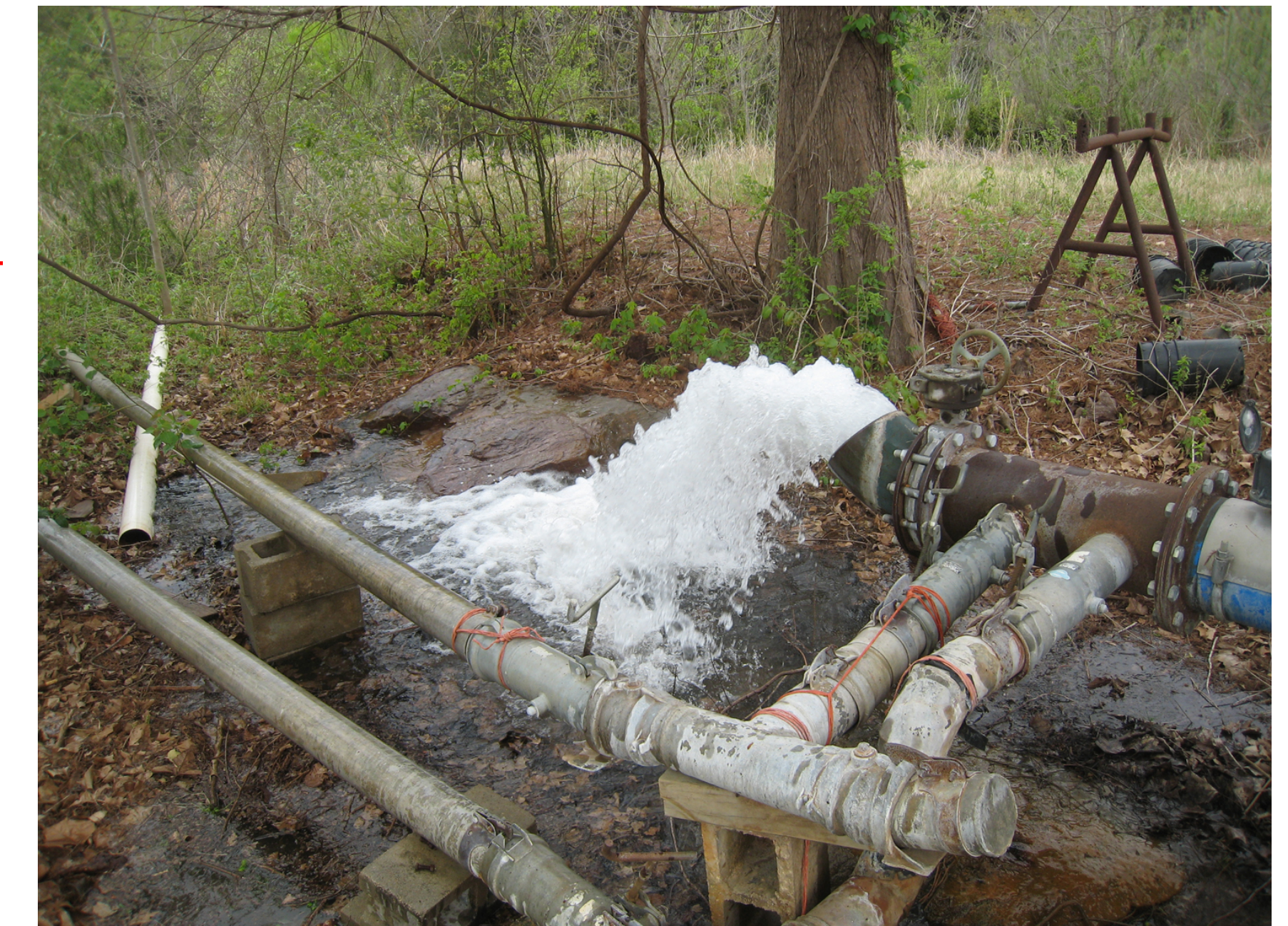
Artesian well near Atascosa, Texas, releasing water from under confining rock units.
