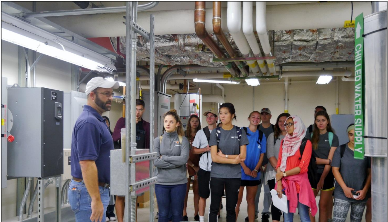
Brian Stokes, mechanical engineer with Facilities Services, discusses building systems with CAEE students during a tour of the Neural and Molecular Science Building (NMS). The tour helps student see the systems they learn about in class.
