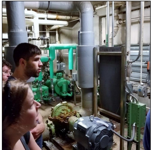
CAEE students get up-close view of UT Austin building systems in operation during facilities tours to support what they learn in class.
