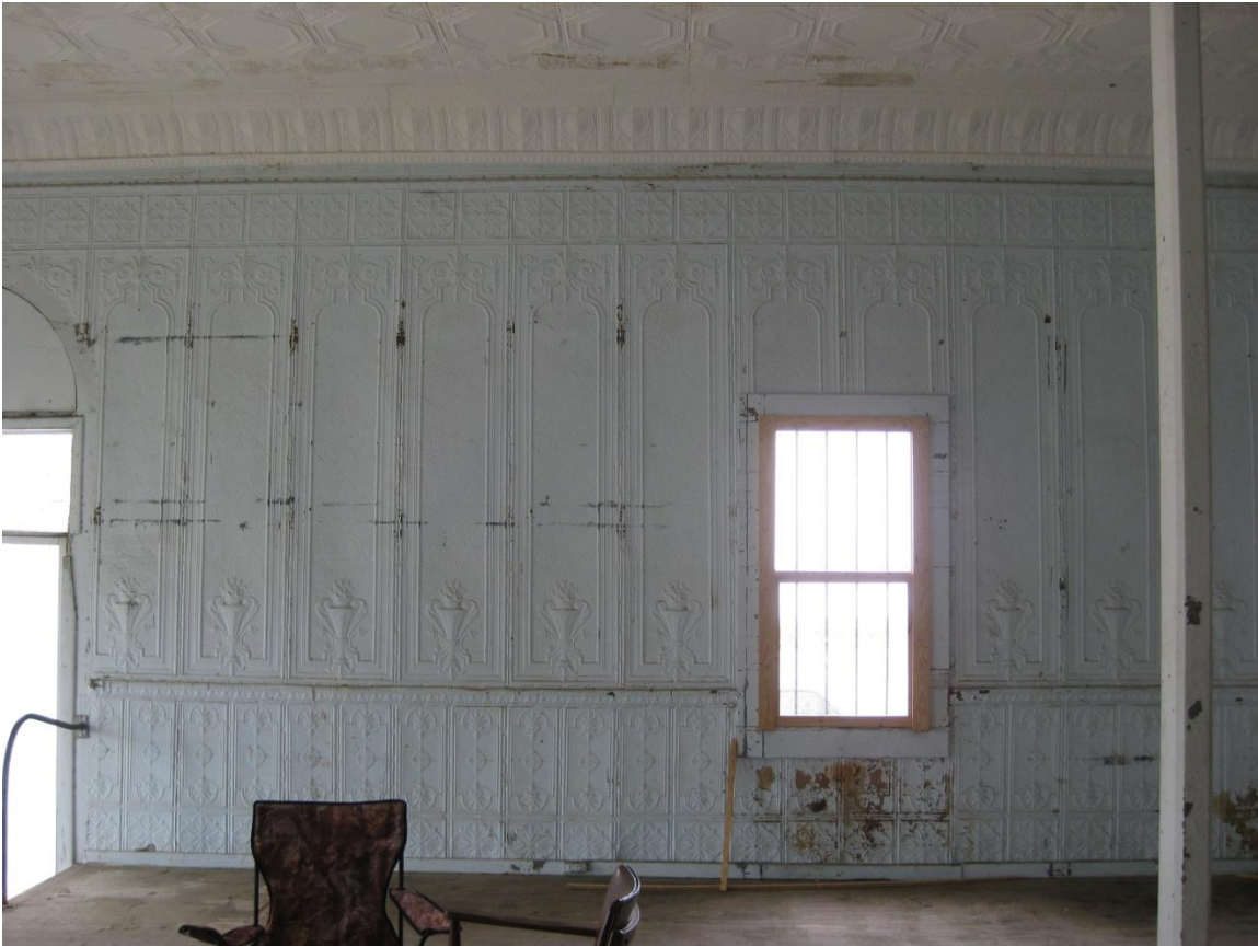
Figure 18: View of southern wall showing pressed metal. Note corrosion under the window.
