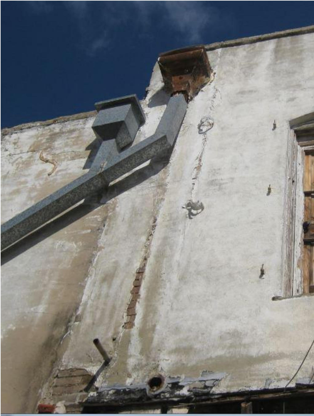
Figure 27: Corroded downspout and stucco loss. West elevation.
