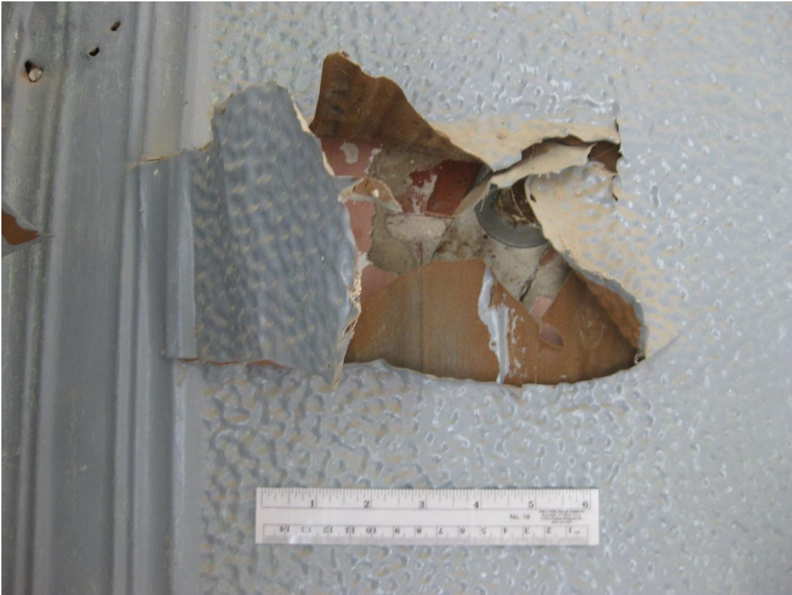
Figure 34: Mechanical damage of the pressed metal wall. South wall.
