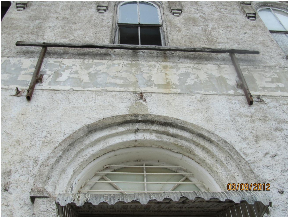
Figure 23: Staining evident on the east elevation.
