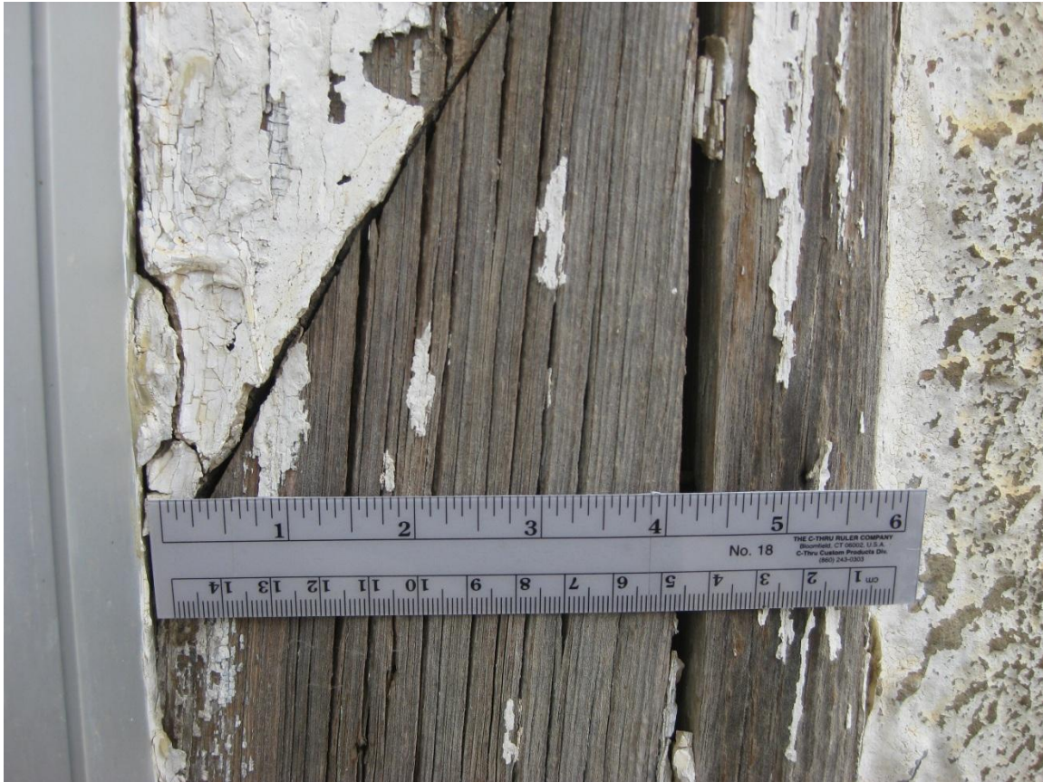
Figure 28: Severely deteriorated wood door frame. South elevation.
