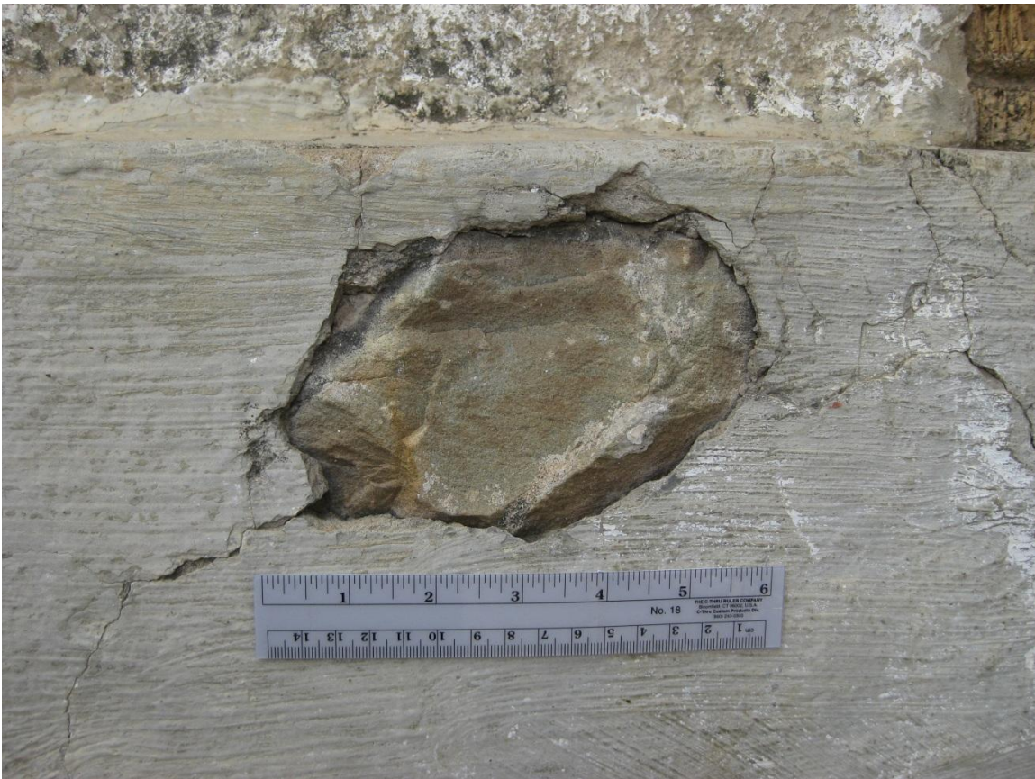
Figure 25: A cement stucco spall from the base of the east elevation.
