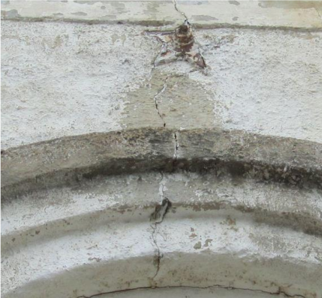
Figure 24: A failed crack patch over the central opening of the east elevation.
