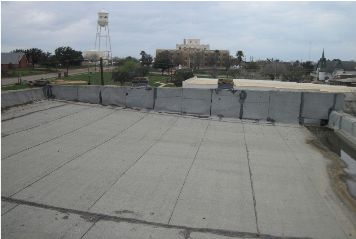
Figure 31: Partial view of the roof with standing water. Camera facing west. (Source: Wade Shoop)
