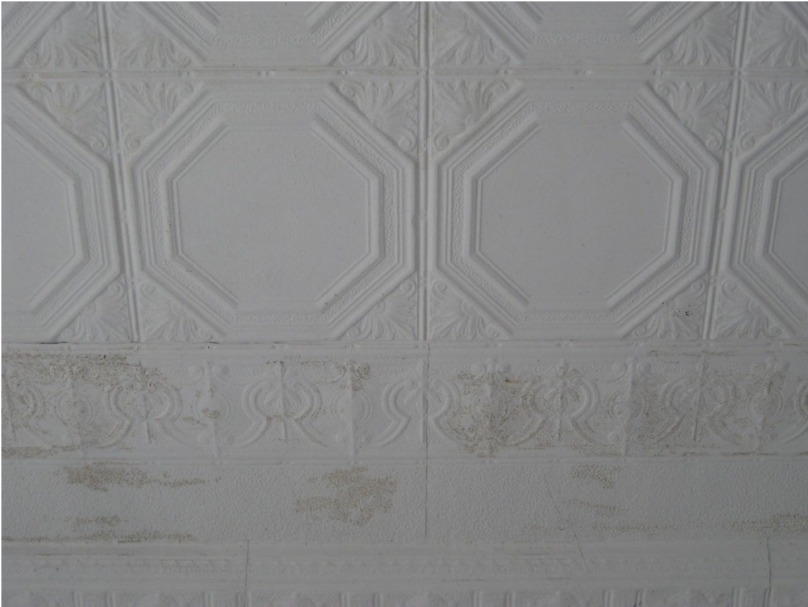
Figure 22: The outer edge of the ceiling's pressed metal. The transitional molding from wall to ceiling is at the bottom of the image.
