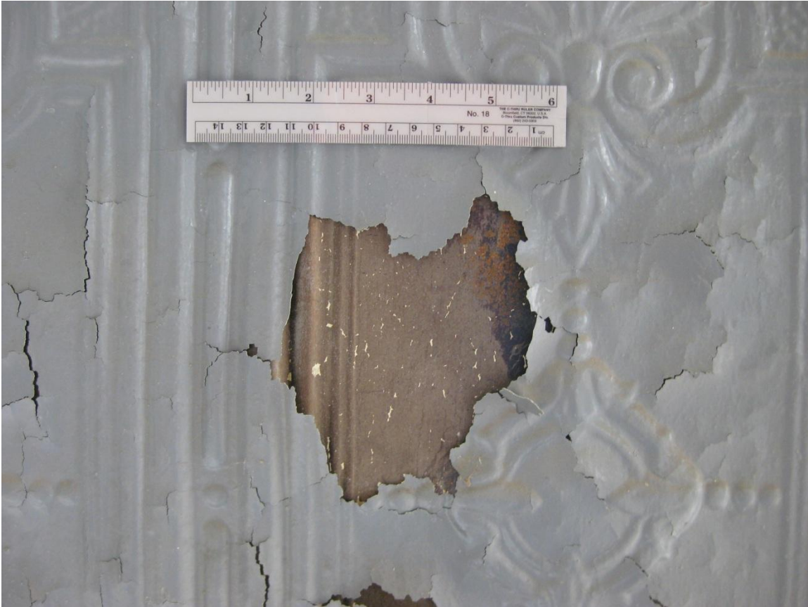
Figure 33: Peeling and flaking paint on the east wall.
