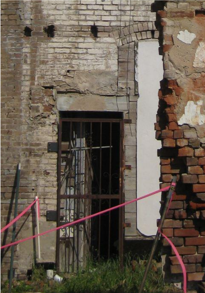
Figure 26: Inappropriate patch, open joints, and holes on the west elevation.
