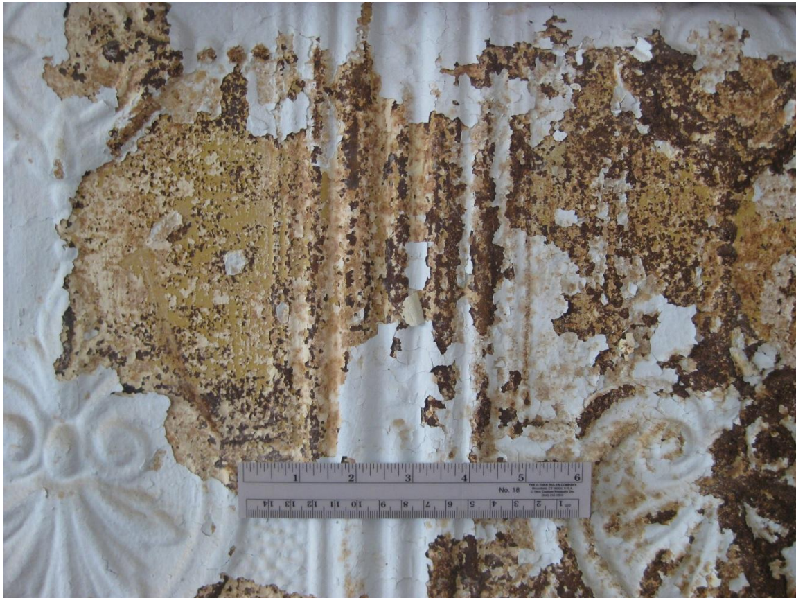
Figure 32: Pressed metal corrosion on the south wall. This area is underneath one the window openings.
