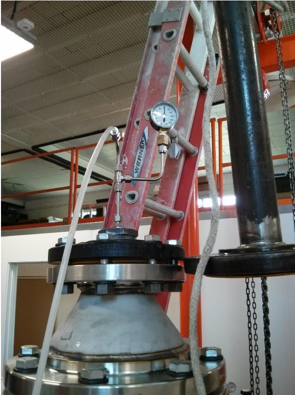
Figure D-2 Air supply and pressure monitoring at the top flange of the chamber
