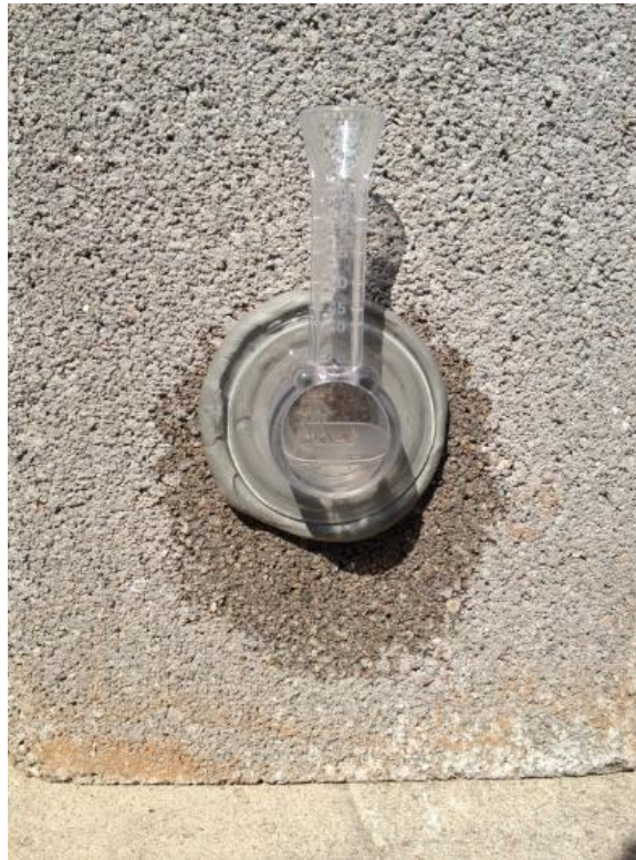
Figure 45: Failed Short RILEM Tube Test on CMU without IWR
