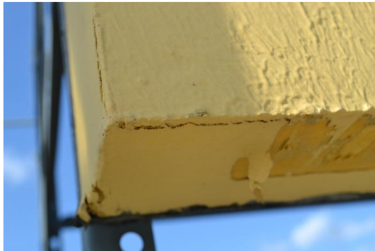
Figure 21: Specimen DRP1009-04 Edge Cracking After 3 Months Exposure
