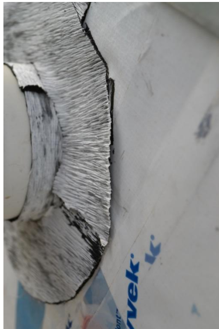
Figure 12: Delamination of Specimen DRP1009-02 Detailing at Large Pipe Penetration After 4 Months—Just Prior to Cladding
