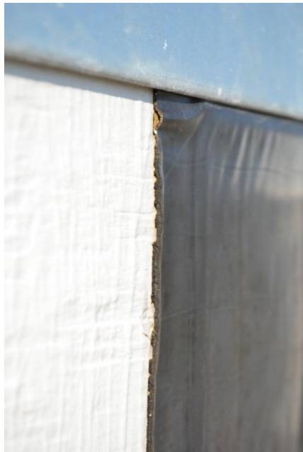
Figure 14: Fishmouthing, Delamination, and Cracking of Specimen DRP1009-05 at Flashing Edge After 10 Months—2 Months Before Required Cladding
