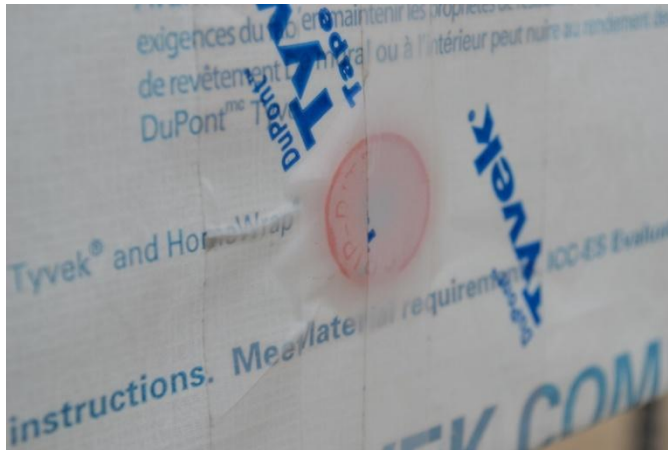
Figure 13: Fishmouthing of Specimen DRP1009-02 Tape at Joint After 6 Months—2 Months After Required Cladding
