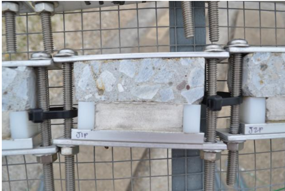
Figure 38: Sealant Specimen DRP1014-J1P (Urethane, SWRI Validated, Primed) Immediately After (top) and 4 Months in Extension (bottom)
