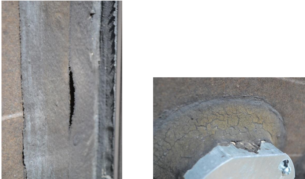
Figure 20: Specimen DRP1009-12 Flashing and Penetration Cracking After 2 Months Exposure
