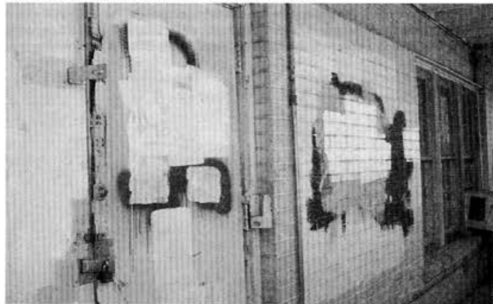
Figure 8. A repeatedly painted-over wall down the alleyway from Mojo's.
