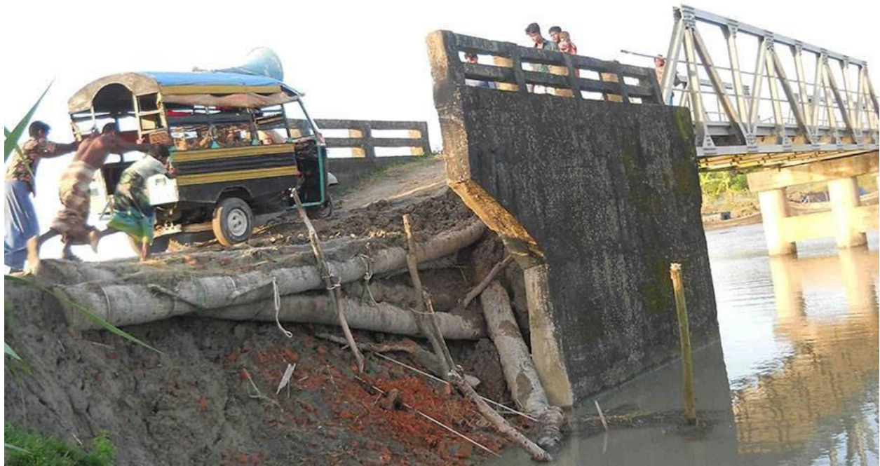
Figure 29 Photograph of a dilapidated bridge between two districts (over Bhulua canal, between Noakhali and Luxmipur districts) do not have fund for repair from either one
