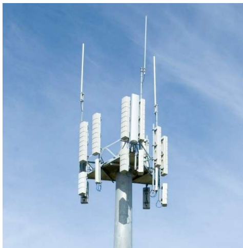
Figure 1.1. Cellular network base station with sector antennas [4].
