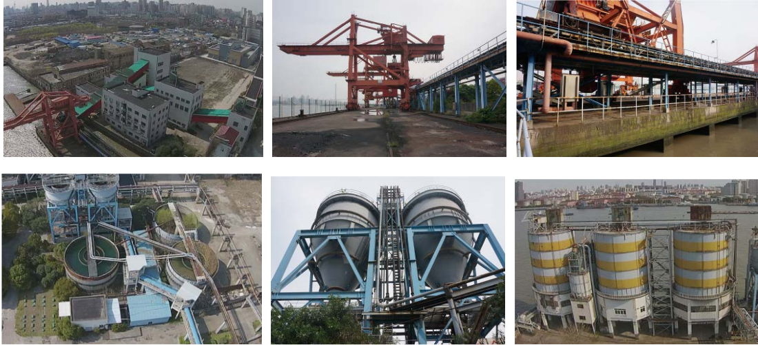
Fig3.19 Coal trestle, terminal crane, conveyor belt, clean water tank, wet ash storage tank, ash storage tank in Power Plant 61
