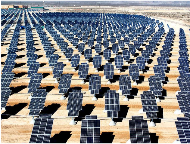
Figure 10.1: Photovoltaic Array, Nellis Air Force Base, Nevada
