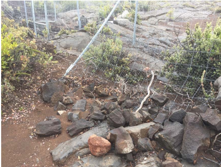
Figure 29 Debris in trap in a wash out area
