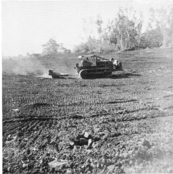
Rolling cleared land. Note how this smooths land surface, making orchard accessible to vehicles.
