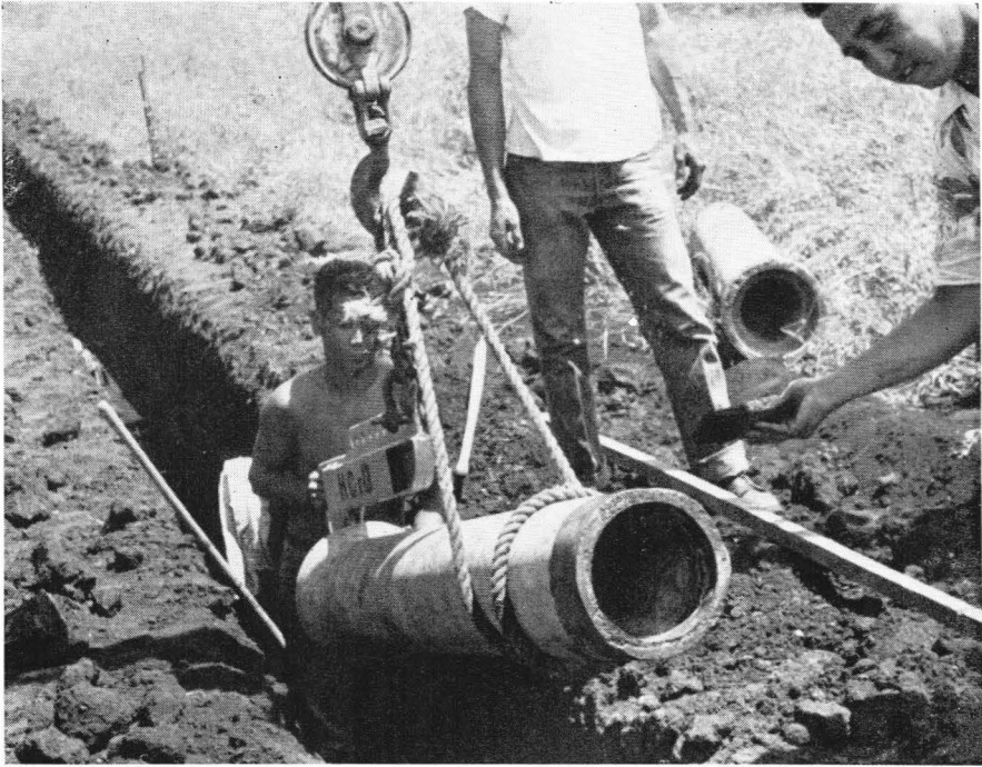
Fig. 42. As the pipe is lowered into the trench by a crane and tongs, the jointing ends are cleaned and wetted by brush.
