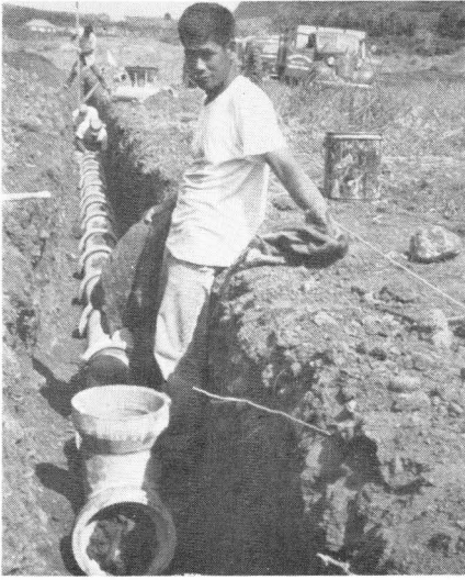
Fig. 26. Risers can be installed by inserting tee-sections in the line. Note burlap in end of pipe to prevent air circulation while the mortar is curing.
