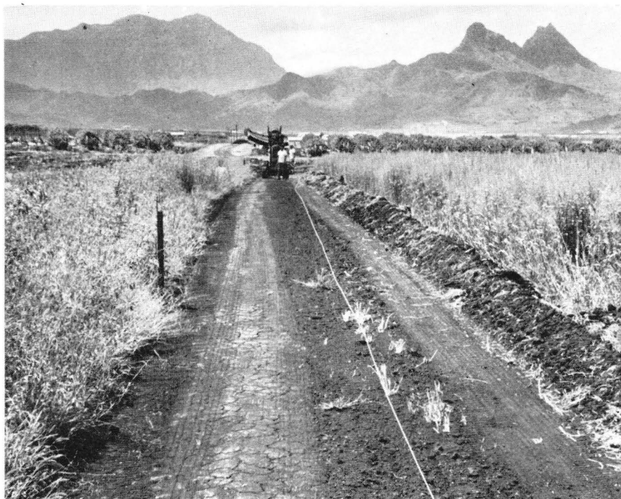
Fig. 38. After insertion of survey stakes (left center), the future site of a concrete pipeline is smoothed by tractor with bulldozer blade. String guides trench digger (in distance).
