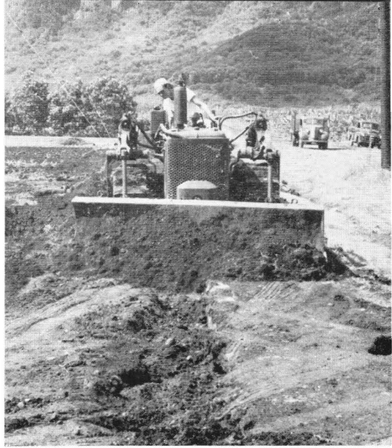
Fig. 48. The final backfilling is done by a tractor with bulldozer blade. Note that the tractor moves across the trench.
