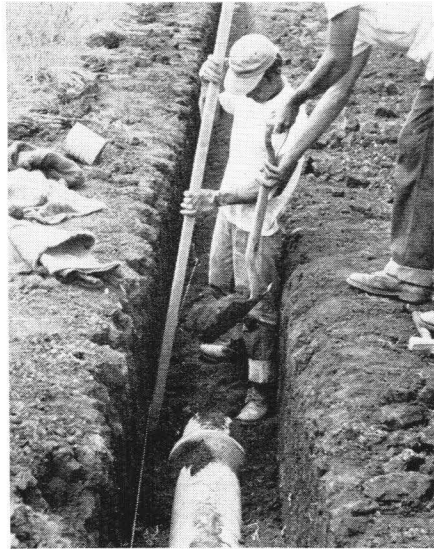
Fig. 46. Moist soil is packed around the pipe and the joint immediately after the mortaring.
