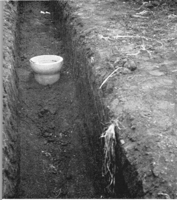
Fig. 47. The initial backfill is done by shovel and is packed well around the pipe by tamping.
