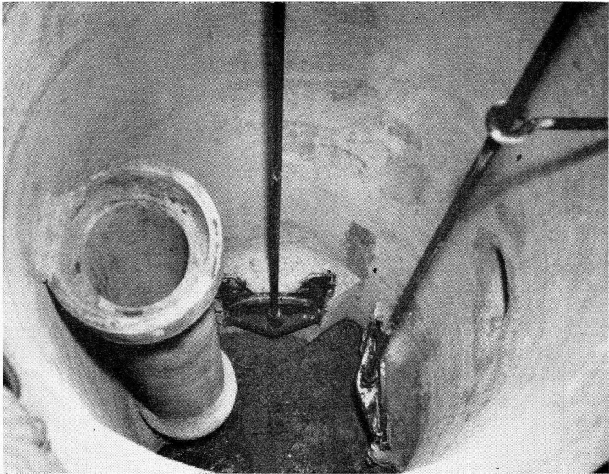
Fig. 12. The inside of this standpipe shows an overflow pipe attached to the upstream inlet (fig. 15d), a surface outlet opposite and below the level of the top of the overflow pipe, and two gates regulating inflow into outlet pipes.
