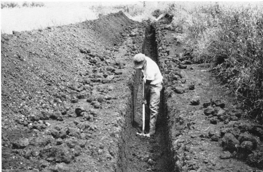
Fig. 40. After trench digging and before checking on the final grade by the trench level, the bed is cleaned by a shovel with a curvature similar to that of the pipe to assure a snug fit of the pipe in the prepared bed.
