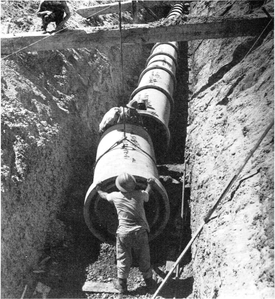
Fig. 9. Flexible rubber-gasket joints are being used in this 36-inch concrete pipe system for sewage conveyance.
