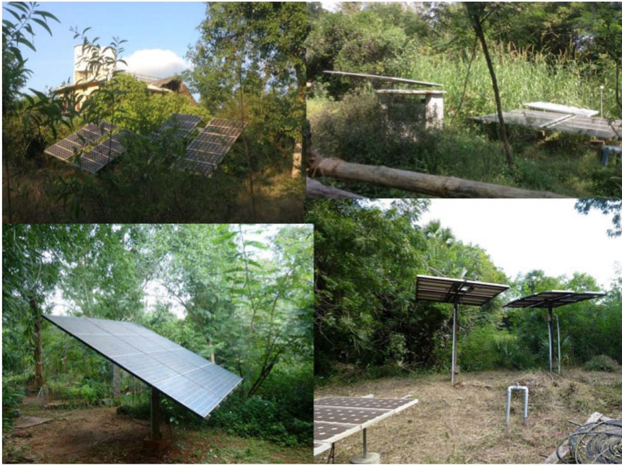
Figure 2: Various photovoltaic installations in Auroville, each affected by forest shading. Note that some installations are far more recent than others and that reasons for shading are complex. In some cases, new arrays were installed with the acceptance of shading to avoid loss of forest; in others, panels were taken down from tall mounts to protect them from storms, and never put back up because the storm damaged the stand. Also, salt corrosion has increased the incentive to keep panels closer to the ground where they can be worked on more easily. Photo by authors.
